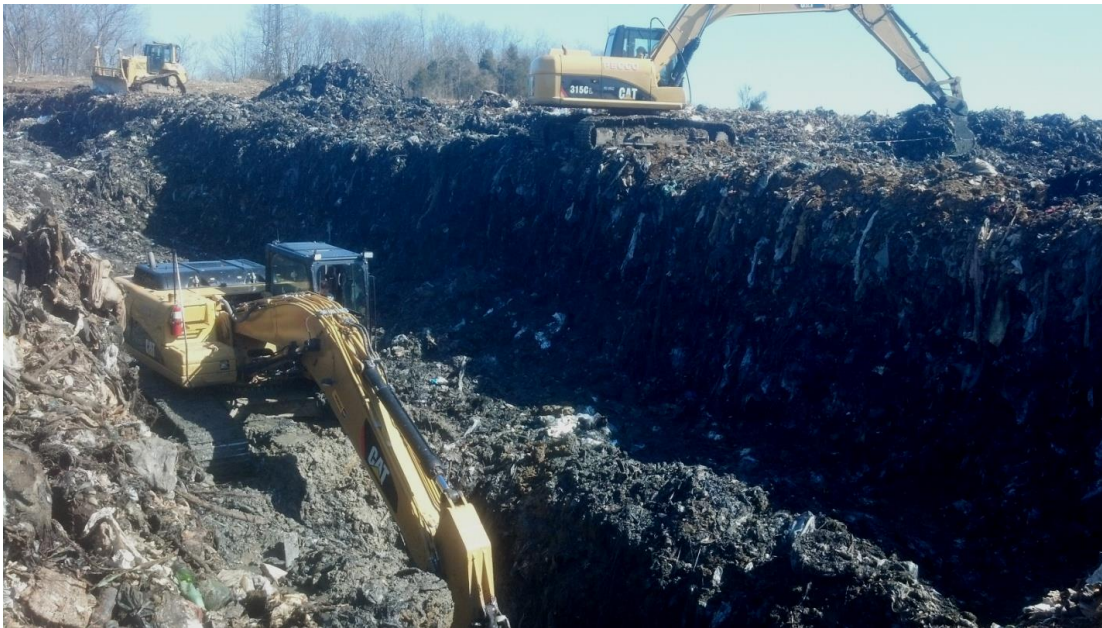
Contractors spent two days digging through trash and rock before uncovering the hidden spring 26 feet below the surface.
