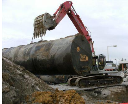
UST removal is taking place at a fueling station. Photo by Division of Waste Management staff.
