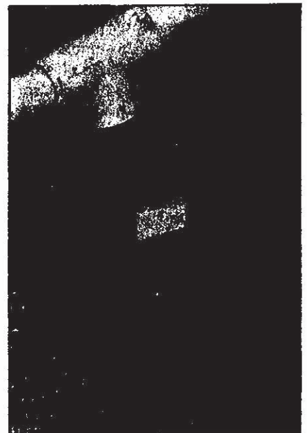
Figure 5. Conductors should be enclosed (top). As shown below the junction box, heavy-duty rubber-covered cord can be used for greater flexibility in installation. All conductors must be of a type recommended for wet locations.
