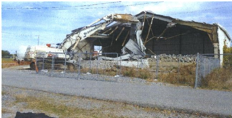
Photo 3: Demolition of former pesticide manufacturing facility. Arkema, Calvert City. Photo by GHD Group Party, Limited.
