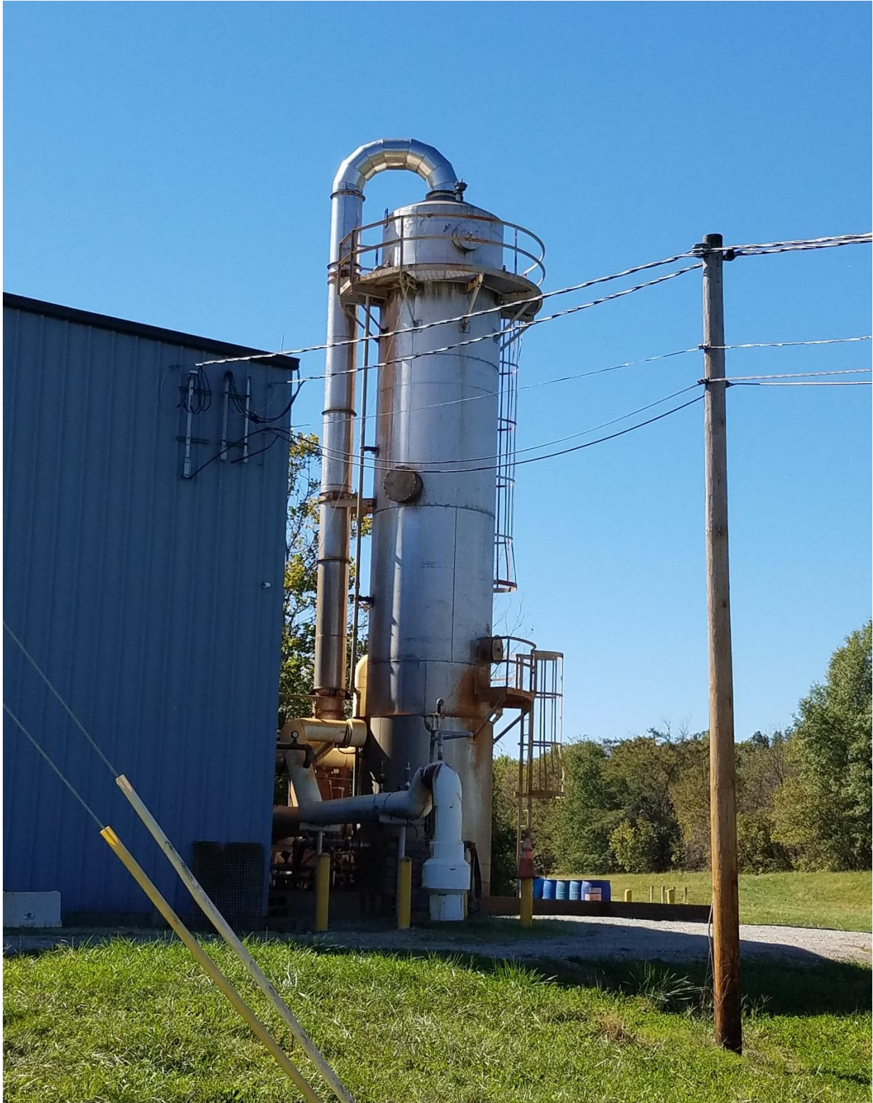
Photo 21 Atkemix Ten Air Stripping Tower, Louisville, KY.
