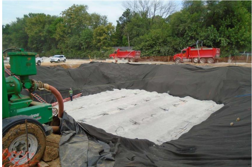
Photo 18: Tank pit area being prepared for installment of USTs. Photo by Rob Staley, Field Office Branch
