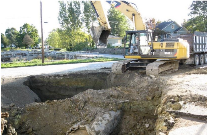
Photo 20: Newly discovered leaking UST. Photo by Rob Staley, Field Office Branch
