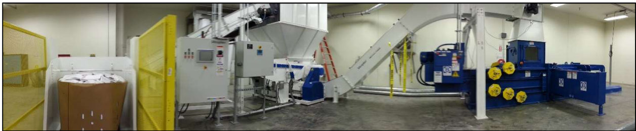
Photo 6: Large Paper Shredder & Bailer at Paper Recycling Section warehouse in Frankfort
