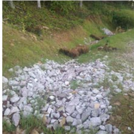
Rock check dams with hay bales in drainage diversion ditch along access road
