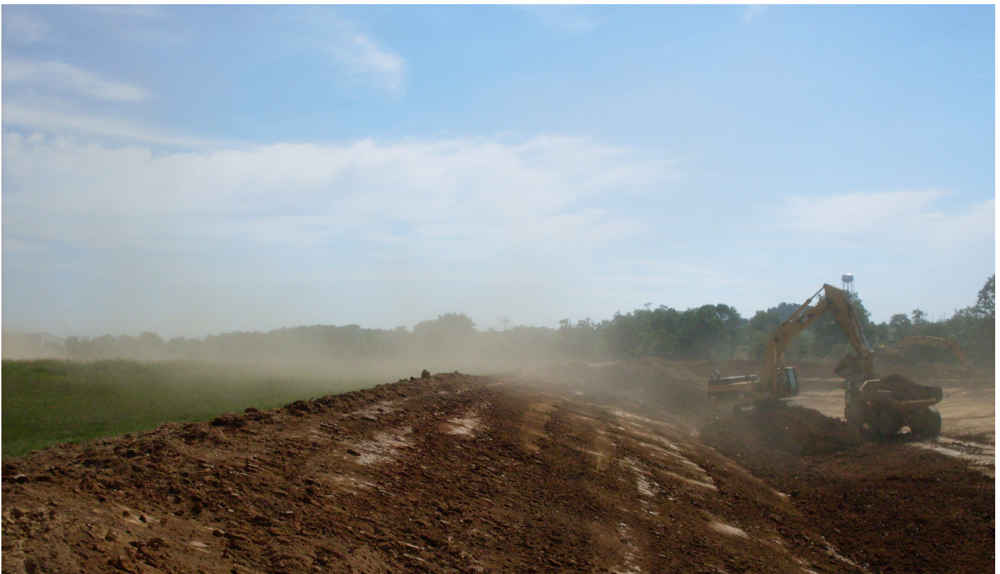
An example of fugitive dust emissions on a construction site. State regulation requires control measures such as spraying with water to reduce fugitive emissions and their impact on air quality. Photo: KY Department for Environmental Protection.
