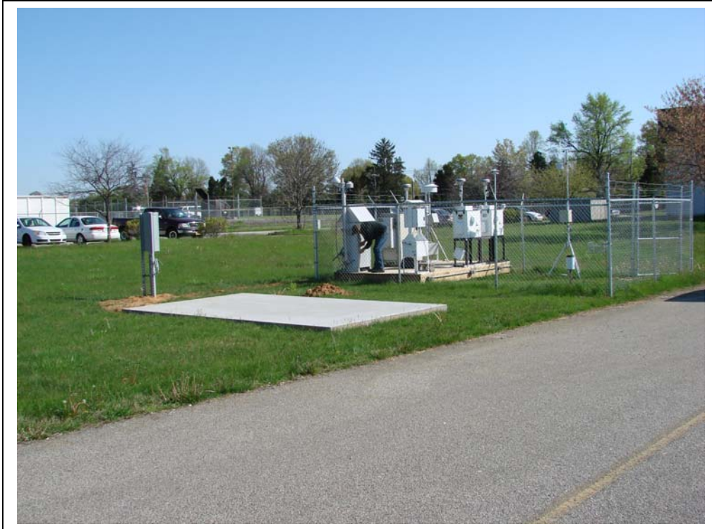
Cannons Lane Ambient Air Monitoring Station
