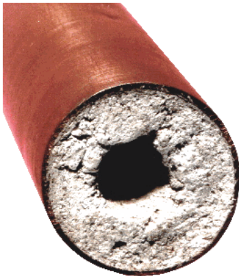
Close-up picture of hard water deposits in copper water pipes.
