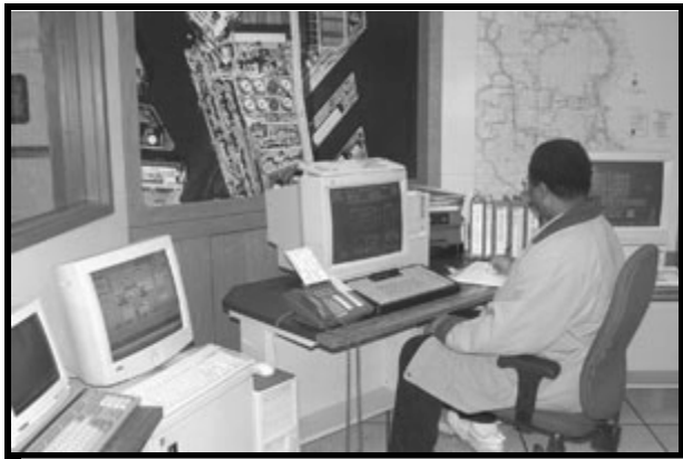
A growing number of sewer systems have shifted to computer-based collection system management [photo: Milwaukee Metropolitan Sewerage District (MMSD)].
