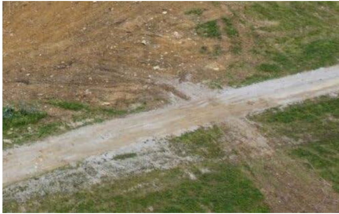
Construction entrance not properly installed
