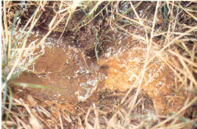
Photo E: Uncontrolled seepage eroding material from downstream slope. Measures must be taken to fill and discharge water in a nonerosive manner.
