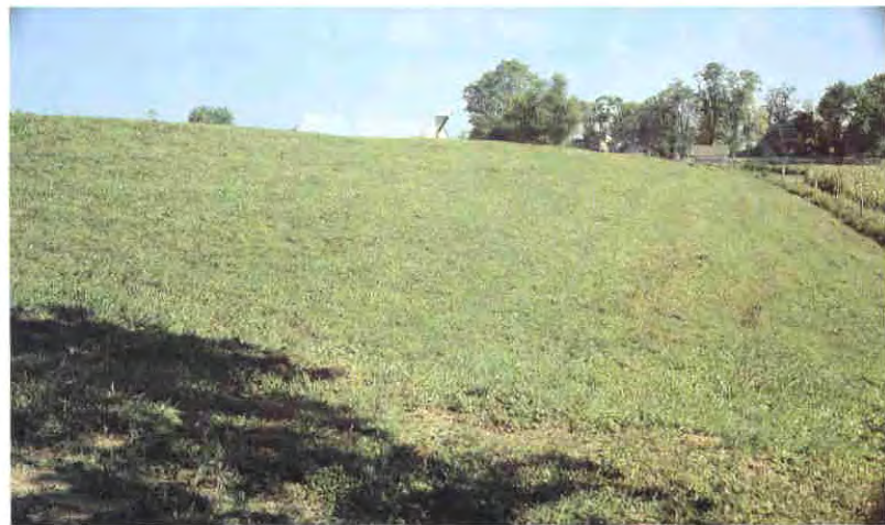
Photo B: Note stand of dense, well mown grass. Inspection will easily reveal any cracks, erosion, seepage, etc.
