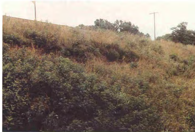
Photo M: Slump on downstream slope. Repair will be a major reconstructive effort. Maintenance has been minimal.
