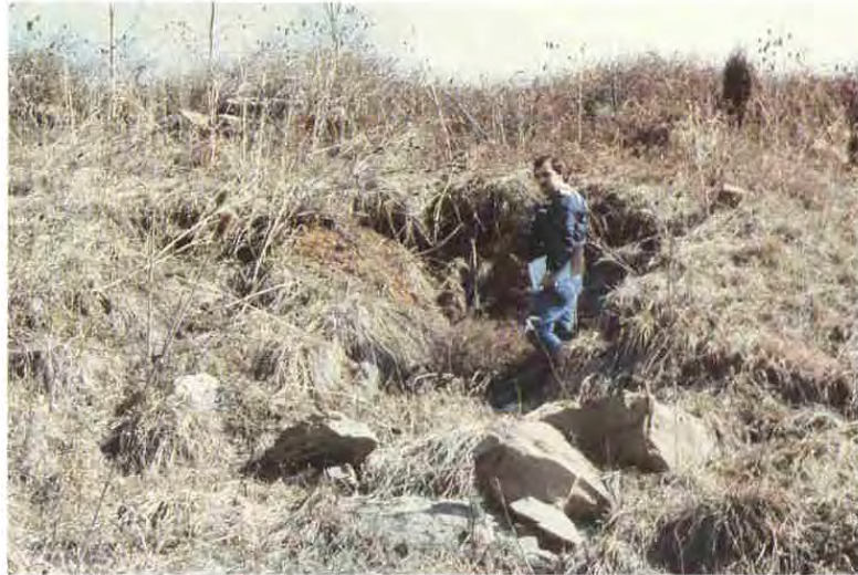
Photo I: Erosion down abutment. Repair will include refilling gully and revegetation.
