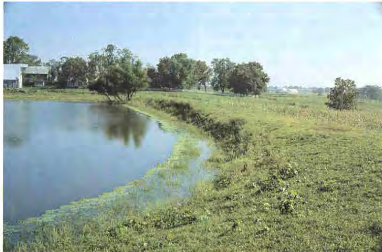
Photo J: Erosion along shoreline due to wave action and water level fluctuation. Maintenance will require some riprap or erosion resistant vegetation.
