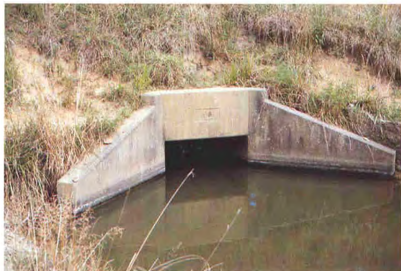
Photo N: Slump on downstream slope. Material has covered drawdown and rendered it inoperable.
