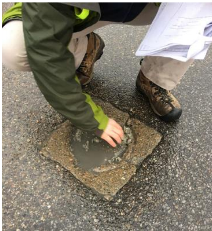
Photo 22: Improper Surface Completion Following a Well Abandonment. Photo by Mitch Hughes.
