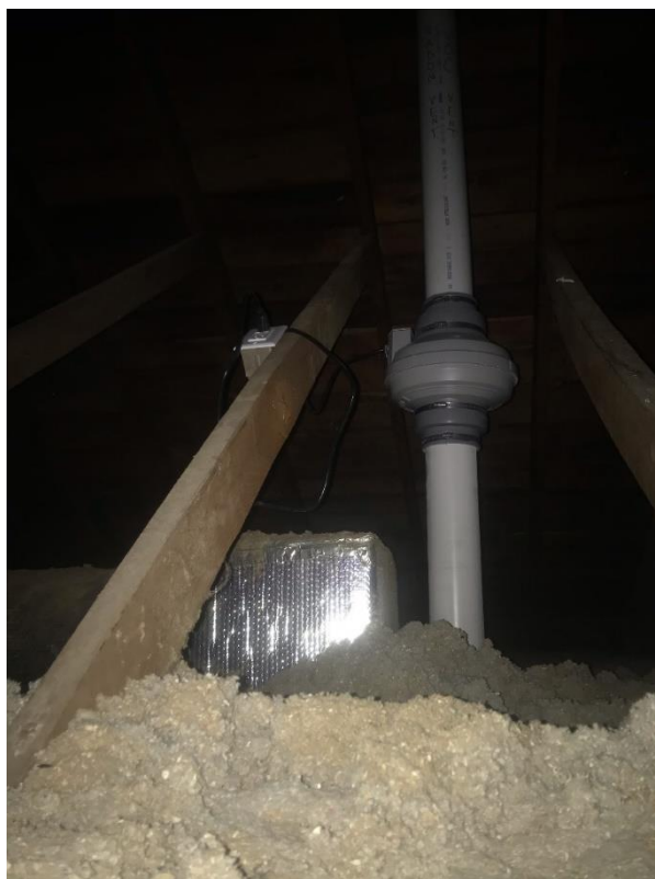
Photo 14: Leitchfield Cleaners Vent Line and Vacuum Routing Vapors Through the Attic. Photo by Chad Von Gruenigen
