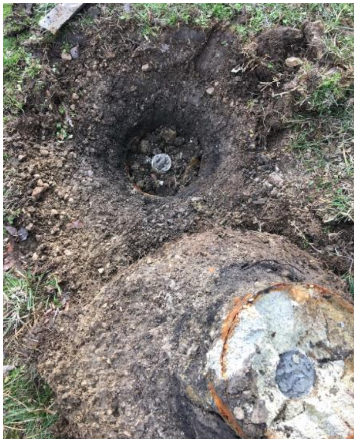
Photo 23: Well Casing, Pad, and Manhole Collar Still in the Ground Following a Well Abandonment. Photo by Mitch Hughes.
