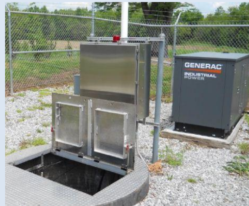
Lawrence Street Lift Station
