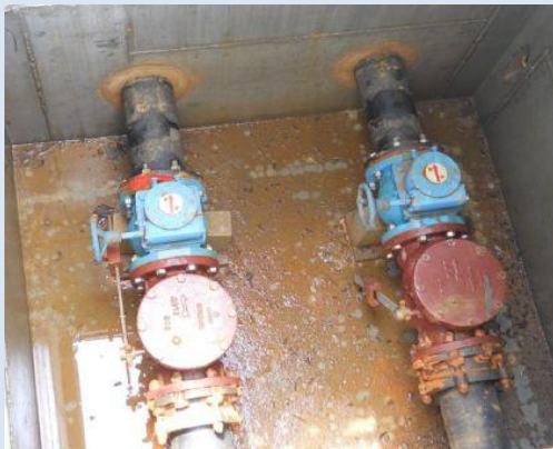
Green Lift Station Valve Vault
