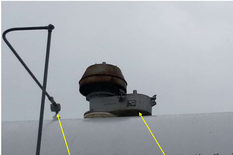
Overfill sensor on top of pentane storage tank
