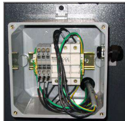
208V & 600V Junction Box
