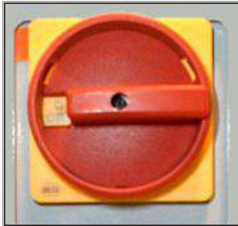
The main power disconnect switch used for safety lockout purposes.
