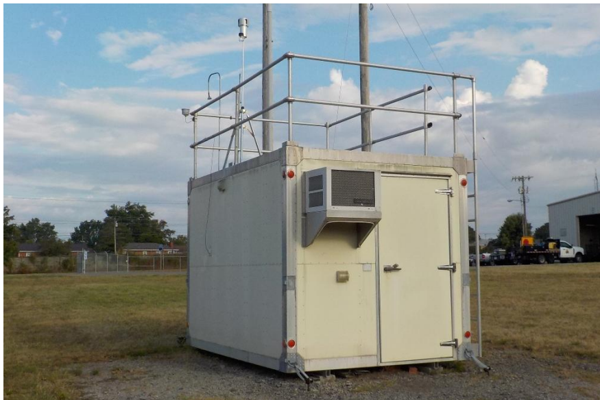
Figure 37: Nicholasville Air Monitoring Shelter
