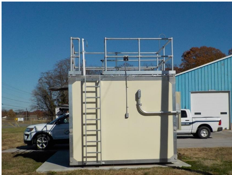
Figure 81: Franklin Air Monitoring Shelter
