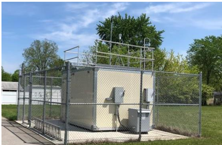
Figure 54: Carrithers Middle School Air Monitoring Shelter
