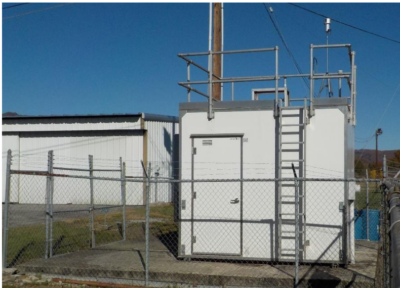
Figure 69: Middlesboro Air Monitoring Shelter
