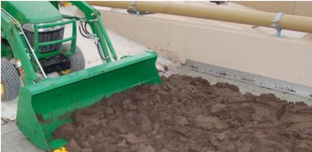
Figure 18.13 Removal of Sludge Cake
