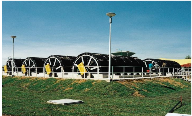
Figure 10.5 Rotating Biological Contactors
