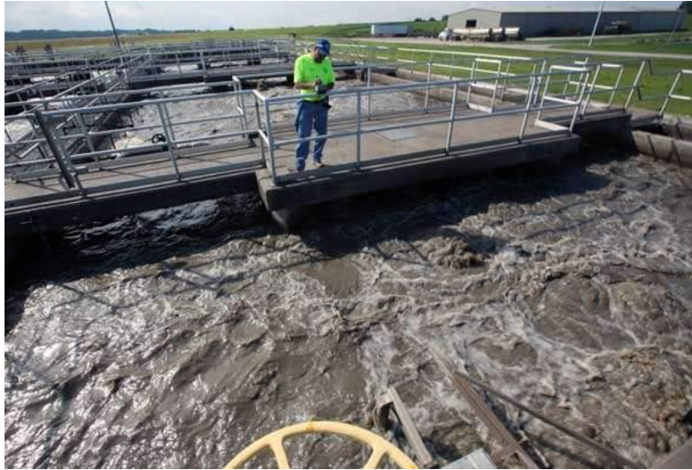
Figure 14.1 Example of an Aeration Basin in an Activated Sludge Process
