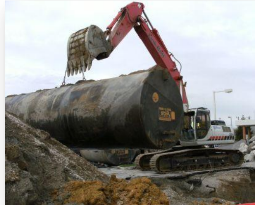
UST removal is taking place at a fueling station. Division of Waste Management staff photo
