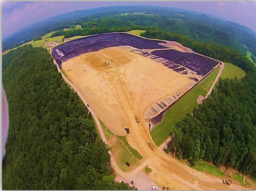
Aerial view of cap construction looking north - photo by Scott Wilburn, MFP, June 2015
