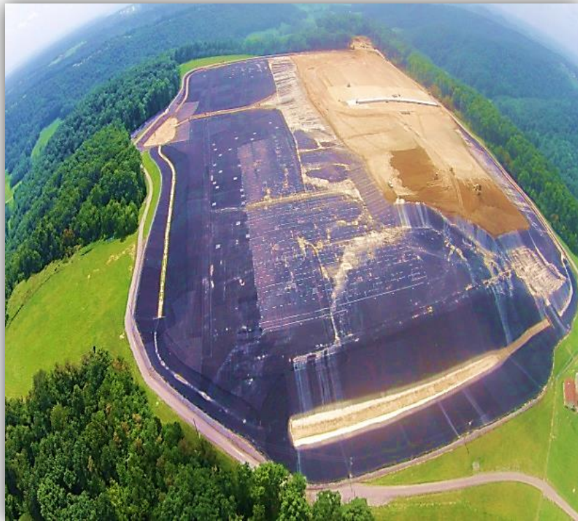
Aerial view of cap construction looking south - photo by Scott Wilburn, MFP, August 2015
