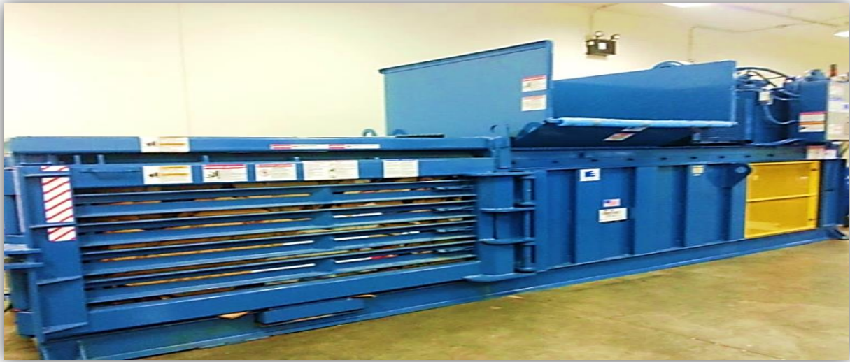
Cardboard Baler at Kentucky Government Recycling Center, Frankfort, KY - photo by Louanna Aldridge, August 2015
