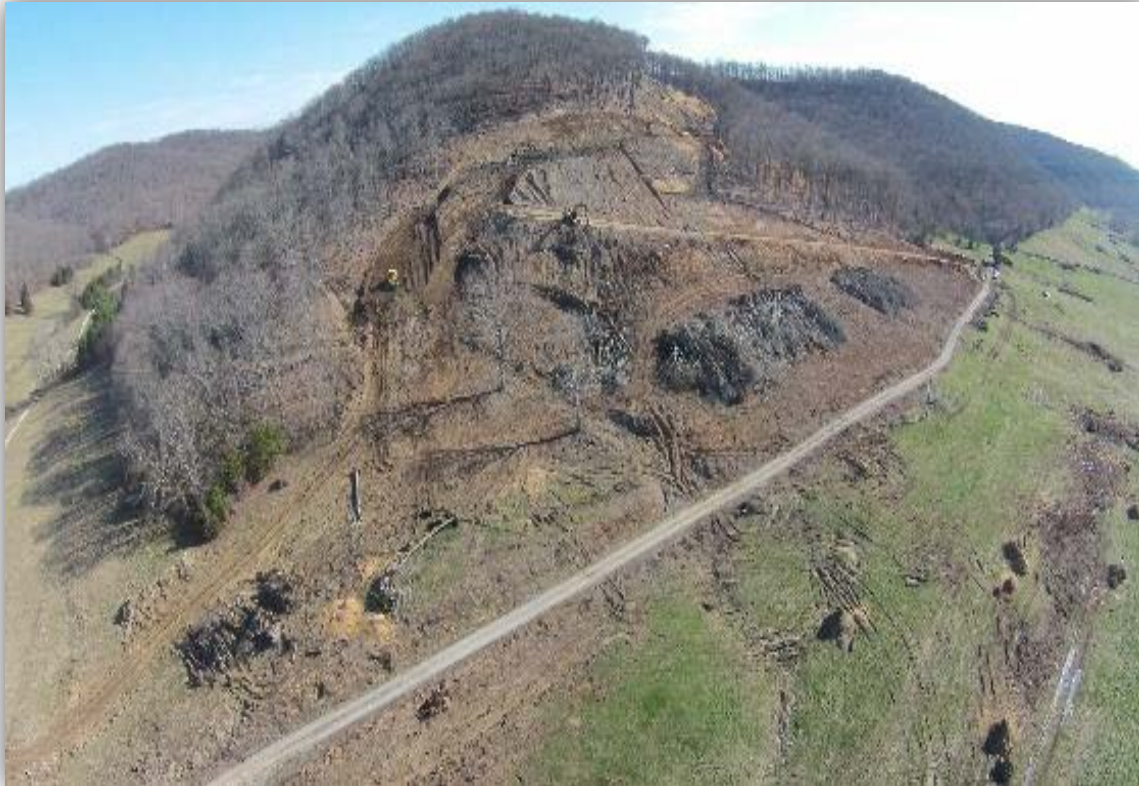
Aerial view of haul road construction - photo by Scott Wilburn, MFP, March 2015
