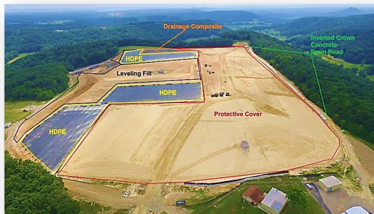
Aerial View of MFP Cap Construction Looking South in June 2016 Photo by Scott Wilburn
