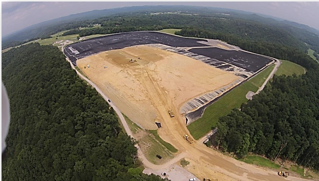
Aerial View of MFP Final Cap Construction Looking Northeast on June 30, 2015 Photo by Scott Wilburn
