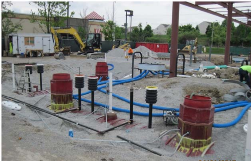
Tank top equipment and product piping installed. Photo by Richard Thomas, UST Branch
