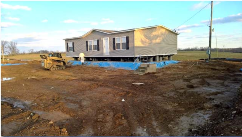
Blue barrier under trailer serving as barrier. Excavations did not occur under trailers on 12/1/16. Photo by DWM Superfund
