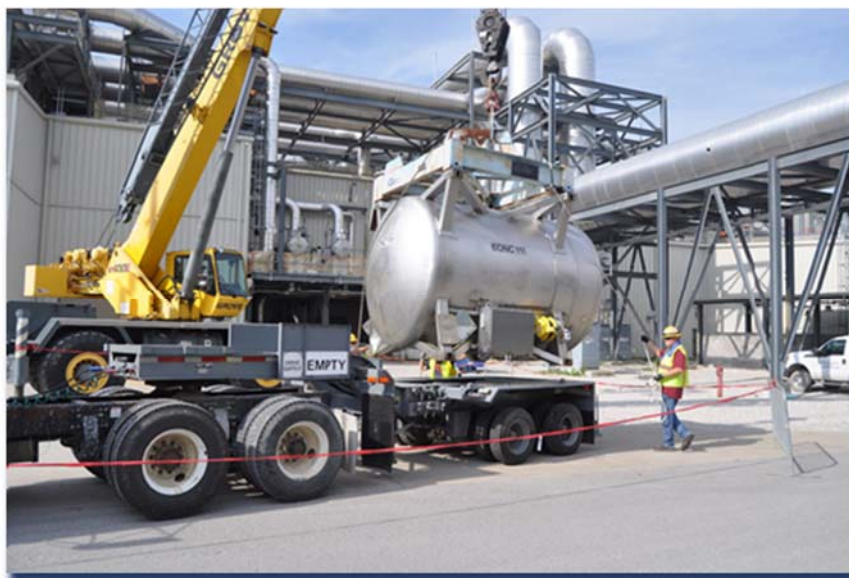
Enhanced on-site container (EONC) practice run. Munitions stored in EONCs for transport from Chemical Limited Area to Container Handling Building. Photo by ACWA.
