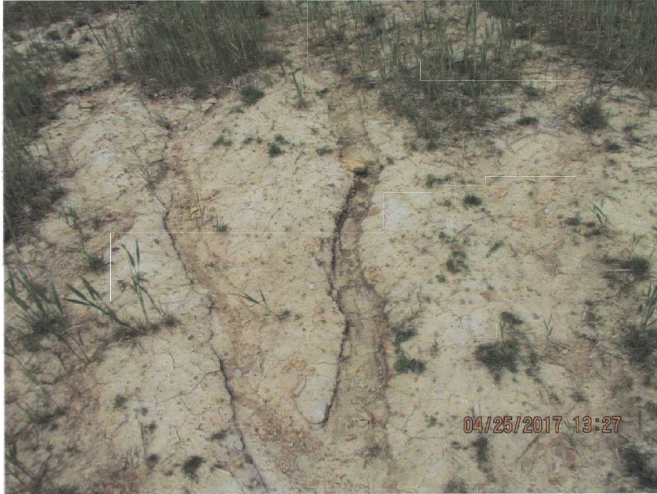
137. Close up of soil erosion/channeling area near the LF monument (the channel is 2 inches deep maximum).
