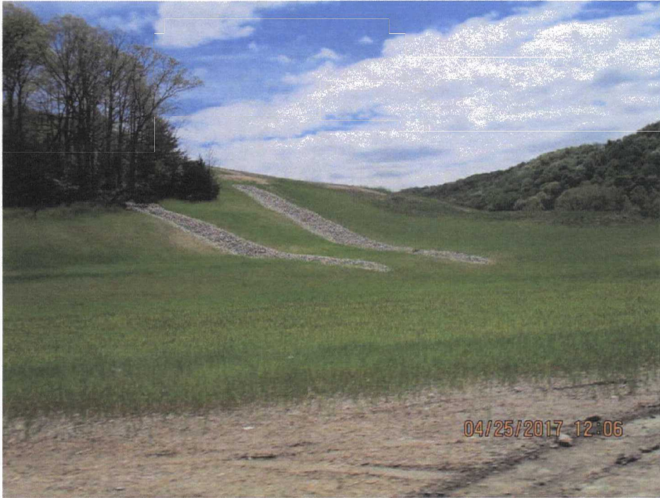
111. Borrow Area #3 where a slip occurred. The slip was repaired and surface drains were installed.
