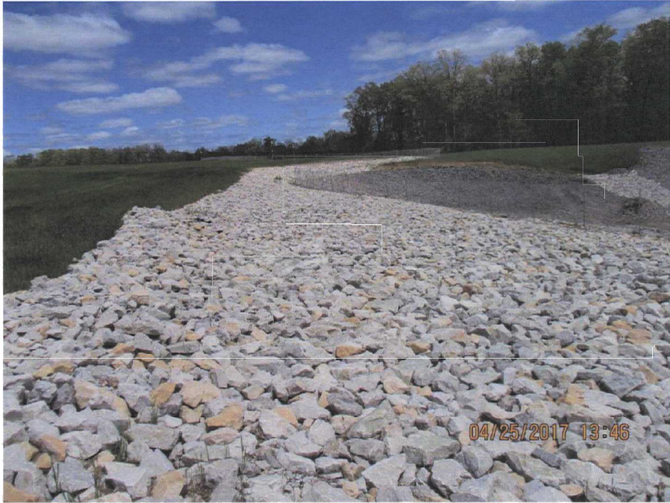
151. Rocks at the edge of the LF cover on the east side of the LF adjacent to the East Basin.
