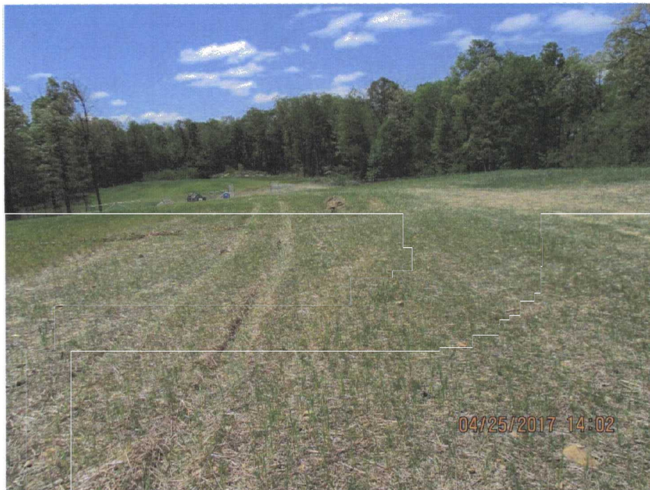
162. Sparse vegetation on the haul road on the LF cap. The southwestern access gate is visible in the distance.
