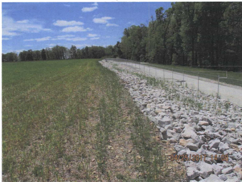
166. Stone at the edge of the LF cap on the south end of the west perimeter.
