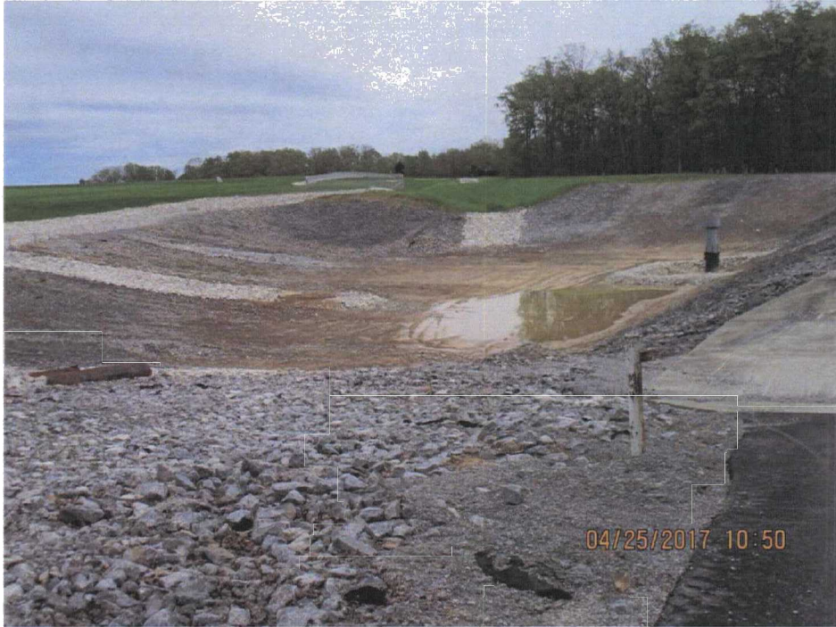
55. Panorama of the east drainage basin from west to north (Photo 2 of 3).
