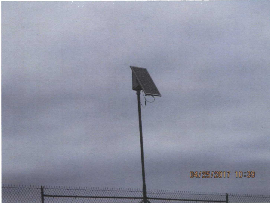
37. Close up of solar panels to power perimeter lighting.
