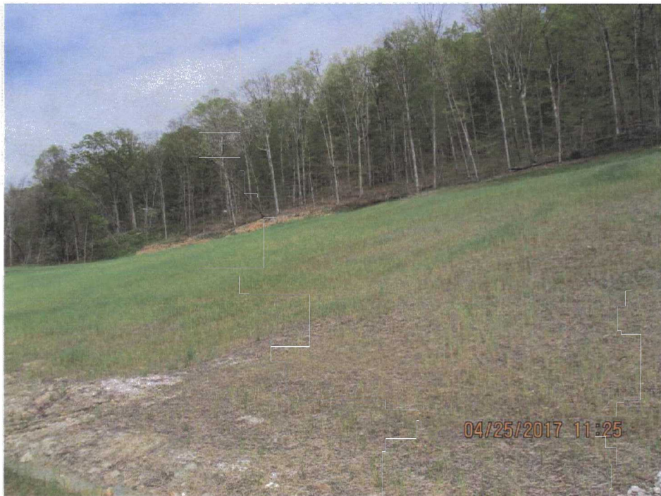
88. Hillside where slip occurred in Borrow Area #4.
