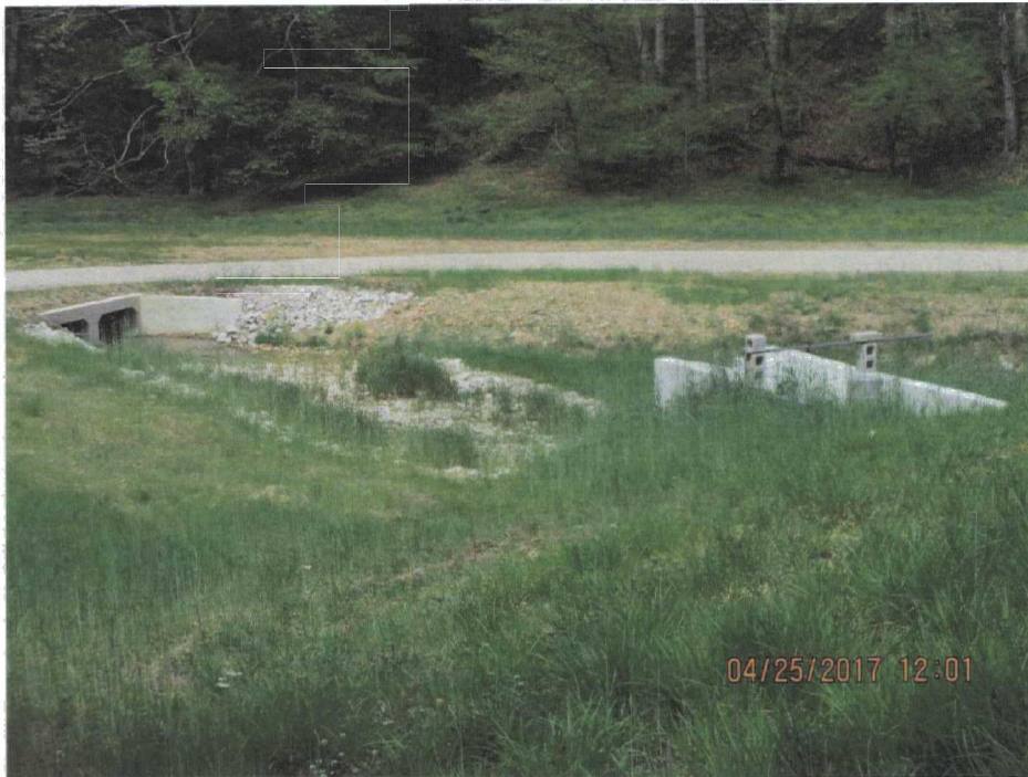
109. Outlet drainage structure from SWMF #3.
