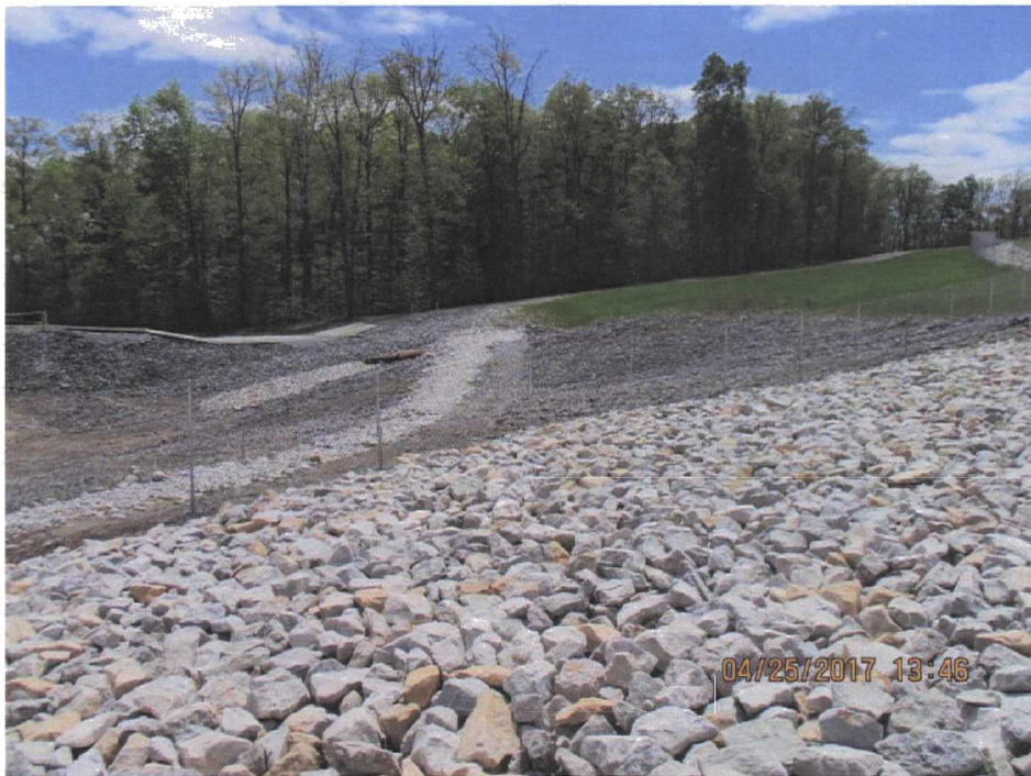
152. Panorama of the east drainage basin from south to north (Photo 1 of 4).
