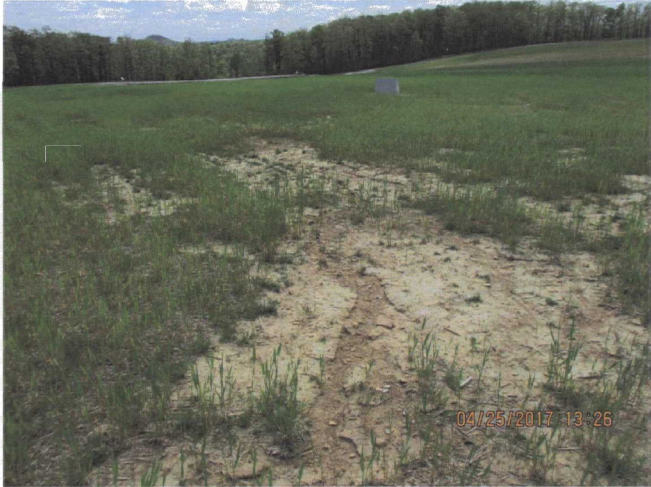
135. A small area with some soil erosion/channeling near the LF monument marker located near the center of the LF.
