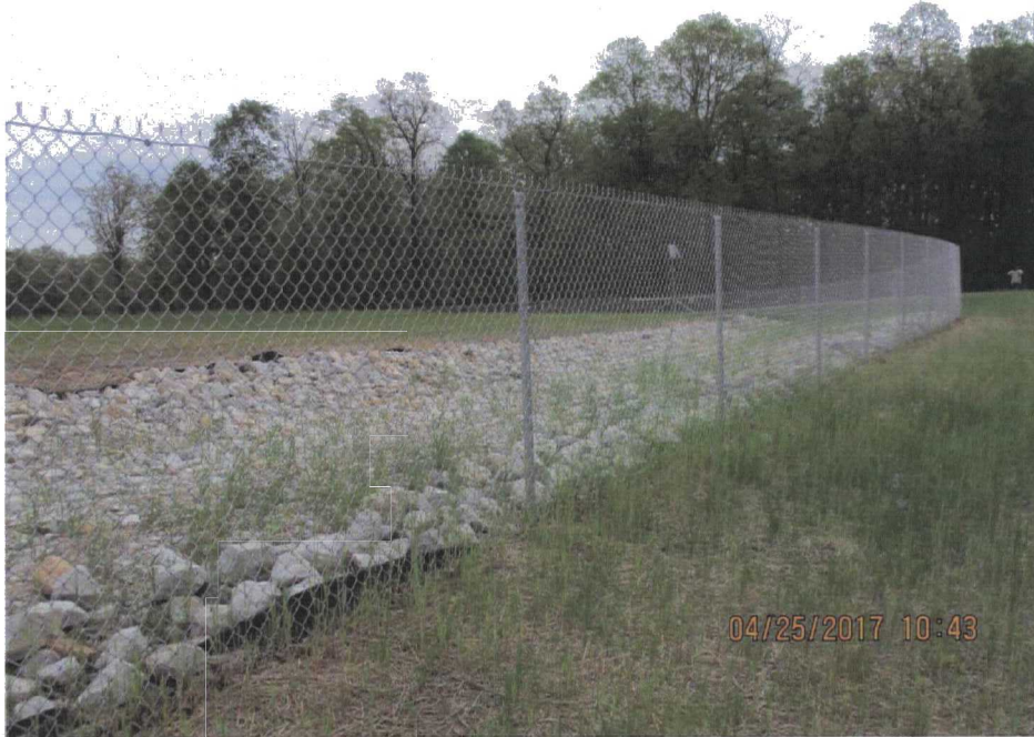
41. Drainage at southeast corner of the LF.
