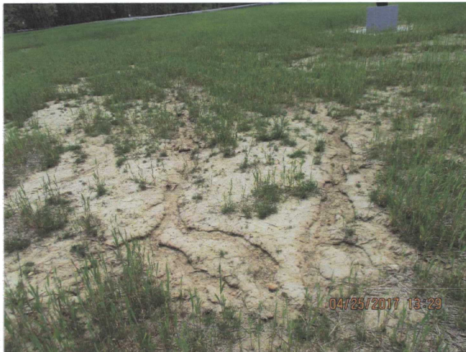
138. More erosion channels that extend towards monument and are downgradient of previous photo location.
