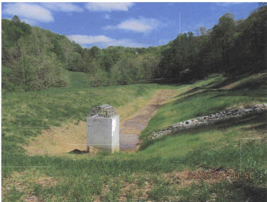
100. SWMF #3 located at the base of the hill on the west side of the LF.
