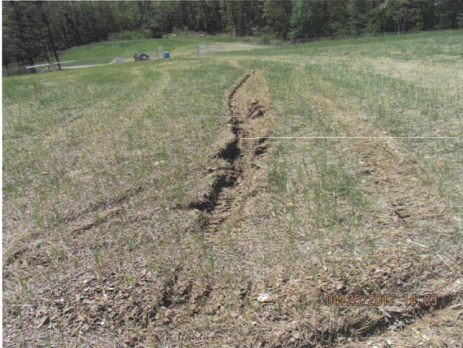
163. Tire ruts in the LF cap near the southwestern access gate.
