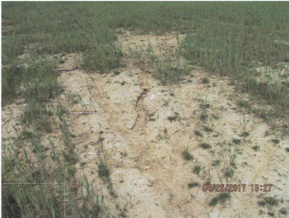
136. A small area with some soil erosion/channeling near the LF monument marker located near the center of the LF.
