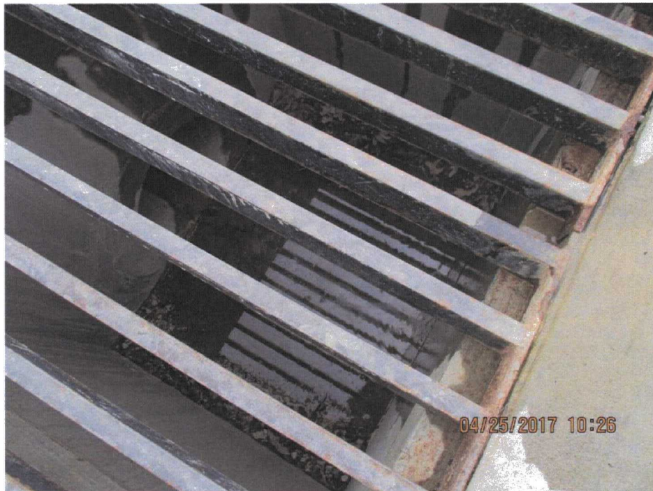
18. Facing down into a storm sump, which provides a break in the drainage direction.
