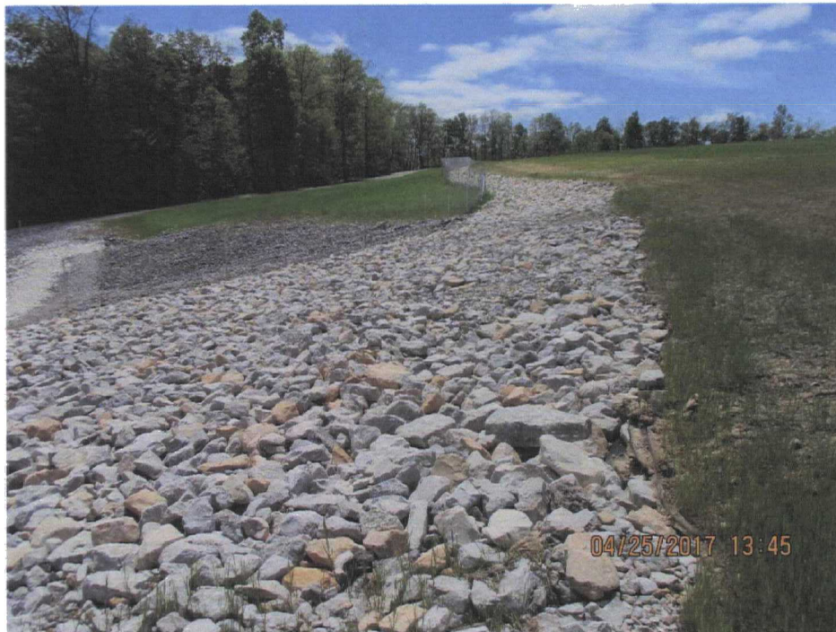
150. Rocks at the edge of the LF cover on the east side of the LF adjacent to the East Basin.
