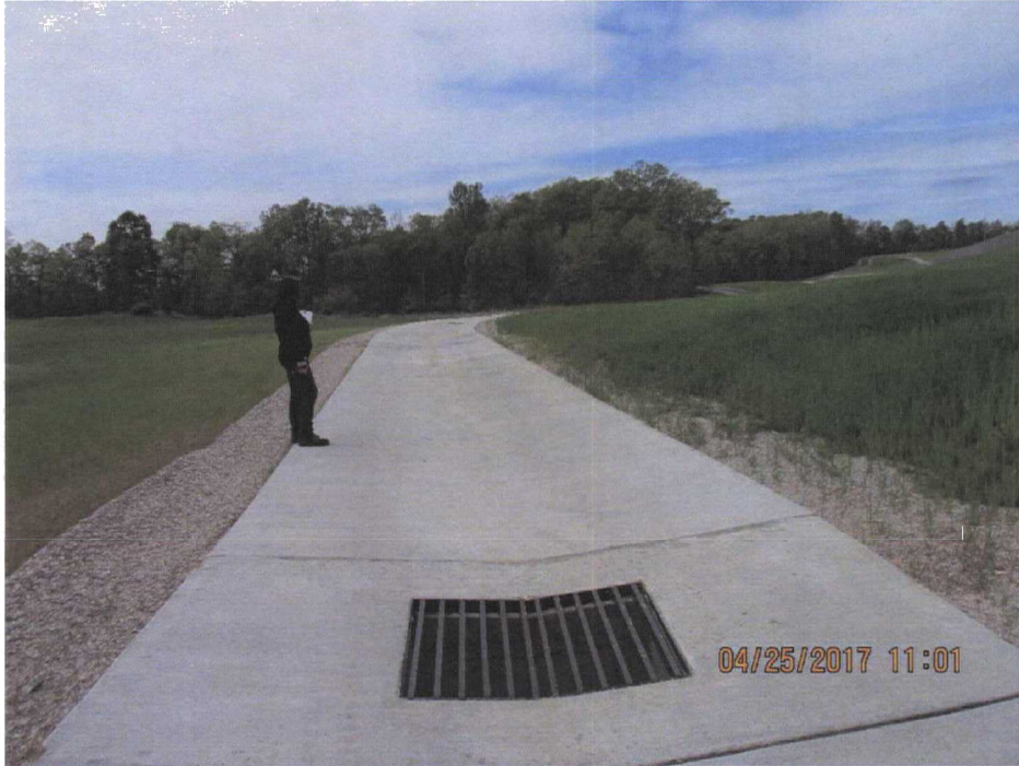
71. Perimeter Road and storm drain near the LF northeastern corner of the LF.
