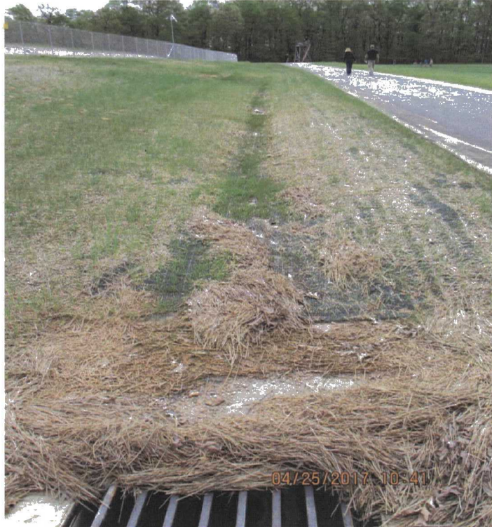
39. Turf reinforcement mat and drainage along the southern perimeter of the LF.
