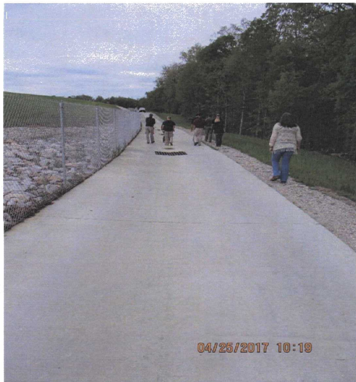
12. Storm drain in the perimeter road in the distance.
