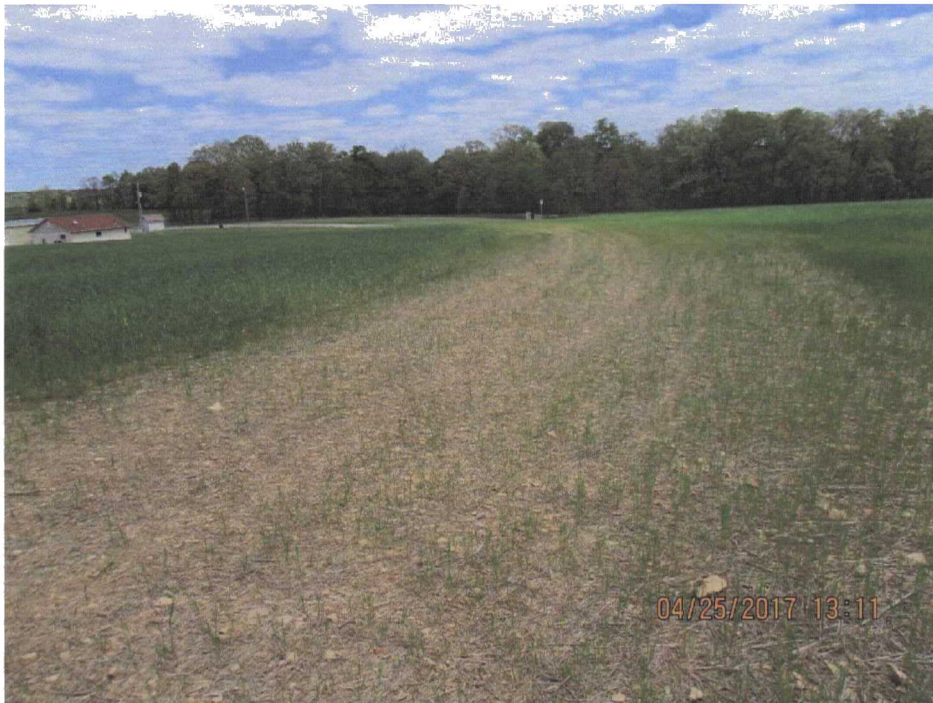
120. Sparse vegetation on the former haul road on the LF cap.
