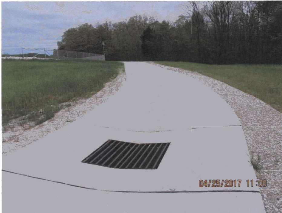
69. Perimeter road and storm drainage near the northeastern corner of the LF.
