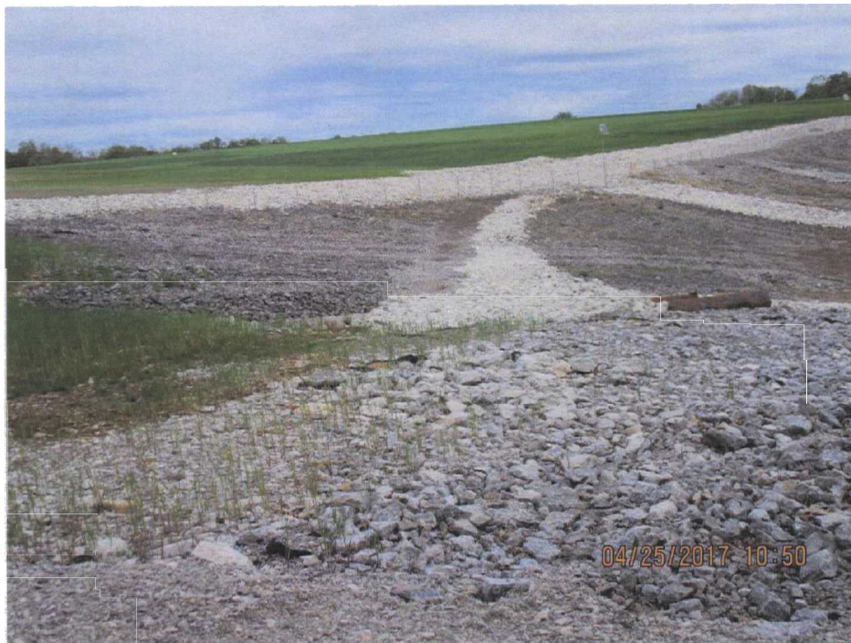
54. Panorama of the east drainage basin from west to north (Photo 1 of 3).
