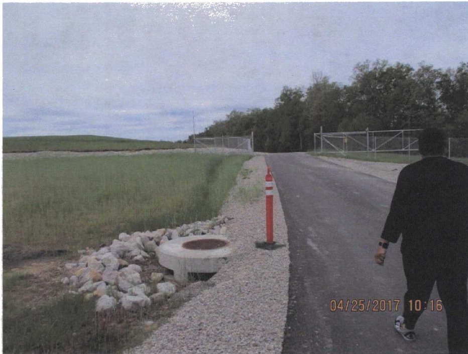
6. Storm drain and culvert to the left and fence and gate to perimeter road in the distance.
