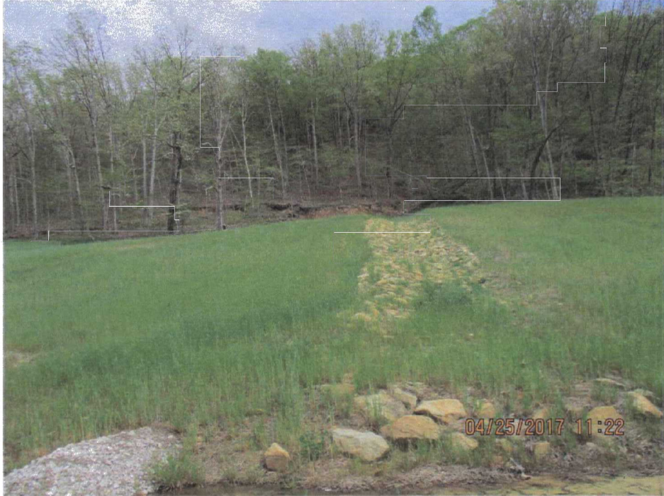
83. A slip on the hillside and constructed drainage in the former Borrow Area #4.
