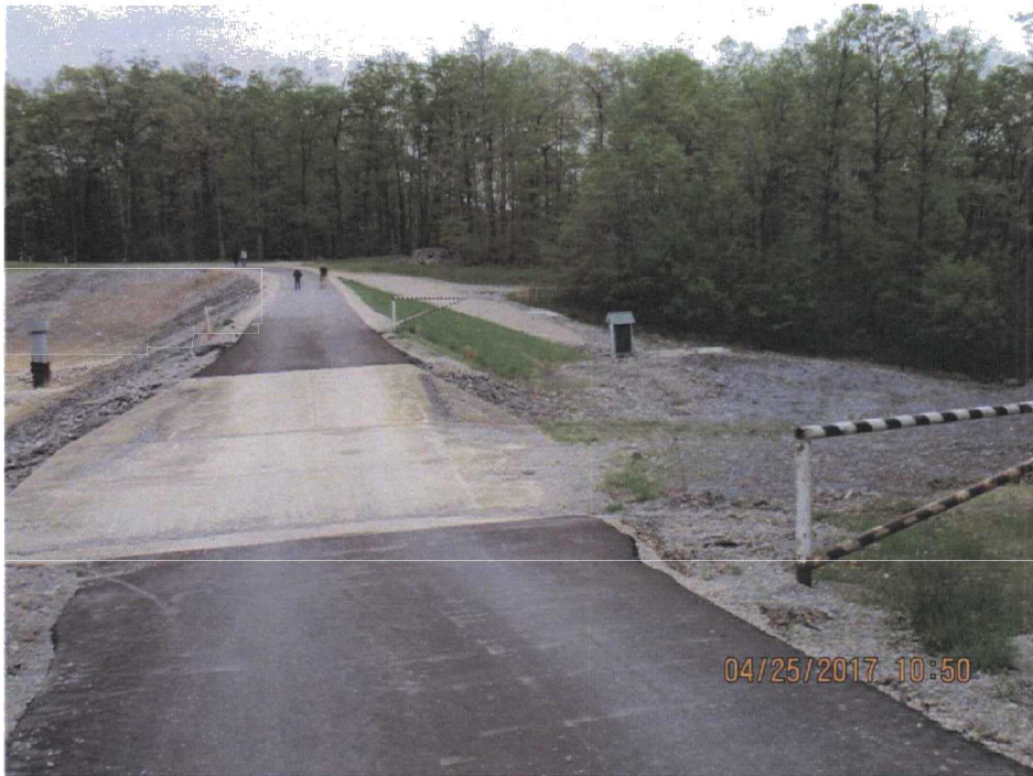
56. Panorama of the east drainage basin from west to north (Photo 3 of 3).
