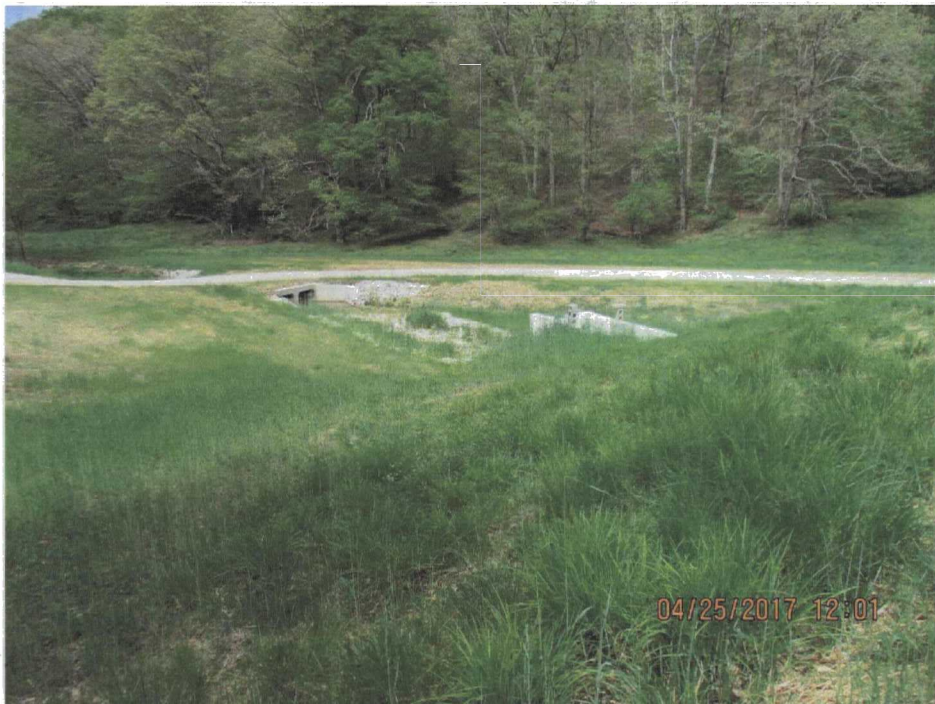
108. Outlet drainage structure from SWMF #3.
