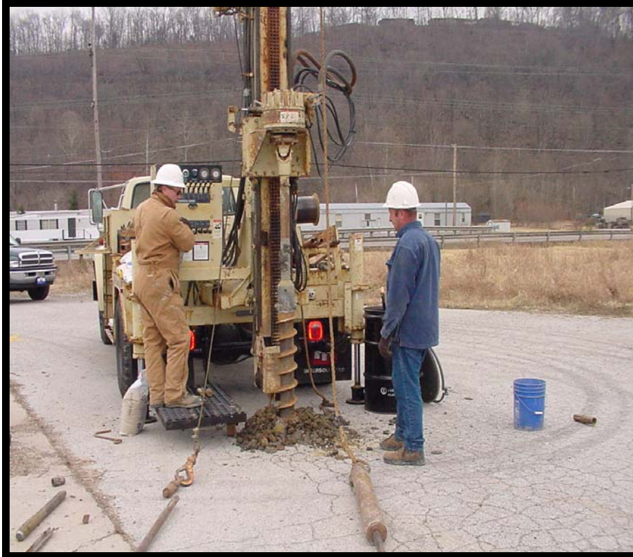
Thanks to Hinkle Contracting for inviting personnel from the Groundwater Branch to observe their monitor well drilling site off Holmes Street in Frankfort, February 7. At left is the certified driller Bobby Roberts, at right is his rig operator Terry McQueen.
