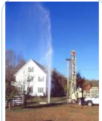
This is not the preferred way to install a geothermal well.
