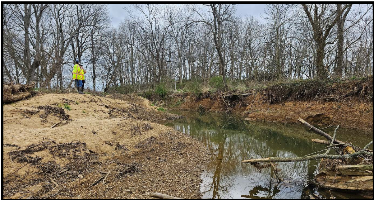
Figure 13. Massive Streambank Erosion in Castleman Creek at Sample Site 12
