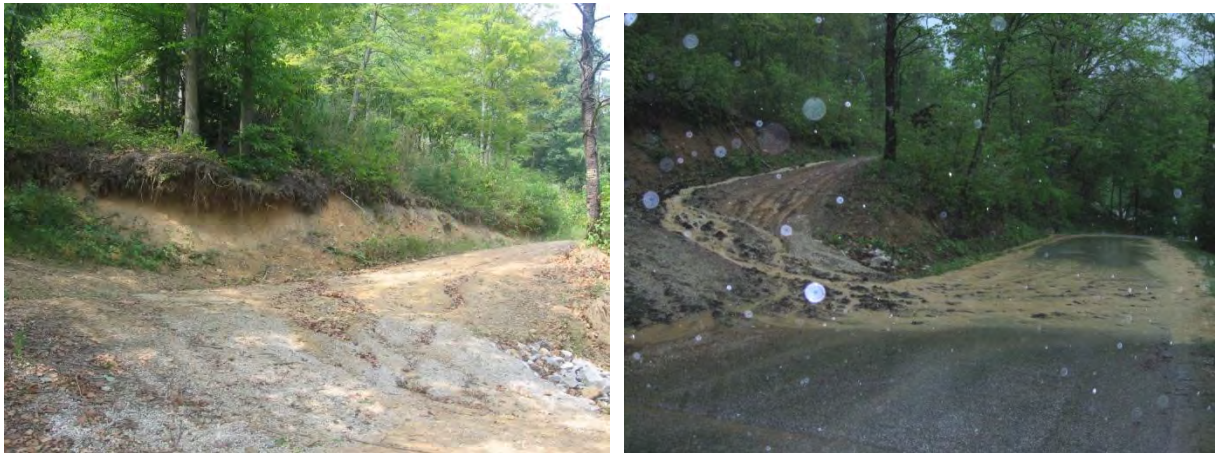
Figure 3.8. An example of poor land use. The photo on the left is a road cut into a hillside. Note the overhanging, eroded bank and gullied road. The photo on the right is the same site during moderate rainfall.
