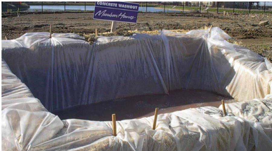
Acceptable containment structure for concrete waste and truck wash water. Make sure that additional structures are available as existing ones are filled.
