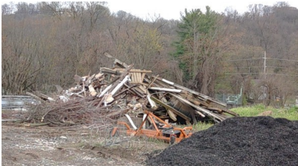
Poor site management of construction debris.
