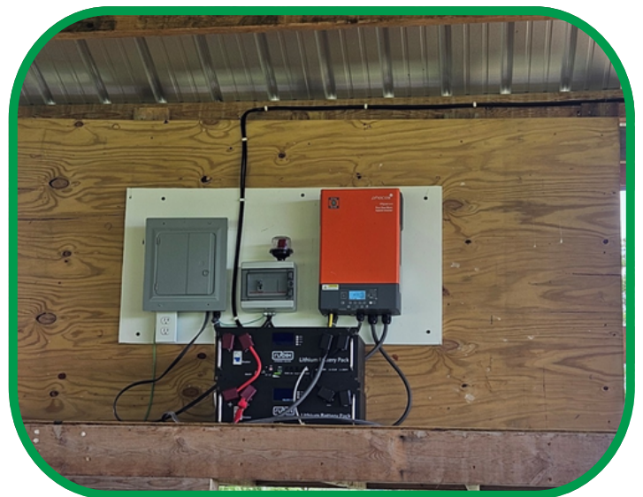
Figure 21: Solar inverter used to power well pumps on a farm in the Bacon Creek Watershed.
