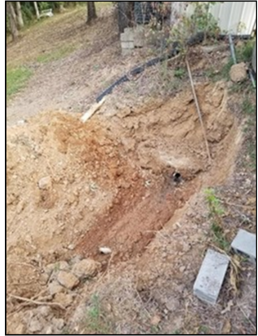
Figure 6. Wastewater straight pipe from a home in the Chestnut Creek watershed.
