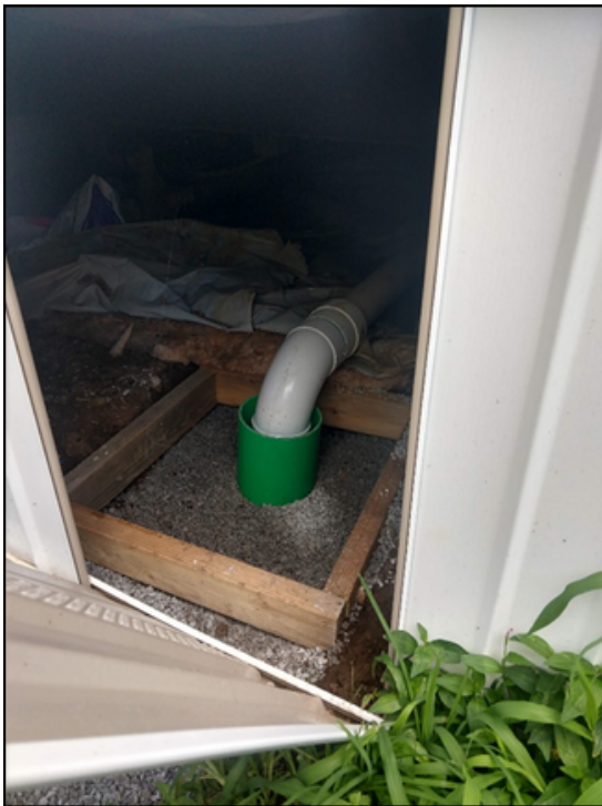
Figure 18. The main sewer line from a mobile home connects to a freshly installed clean-out leading the new sanitary sewer line.
