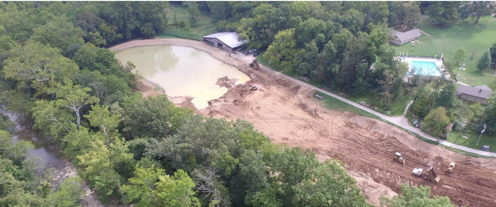
Construction of the bench full wetlands at the YMCA camp near Gunpowder Creek
