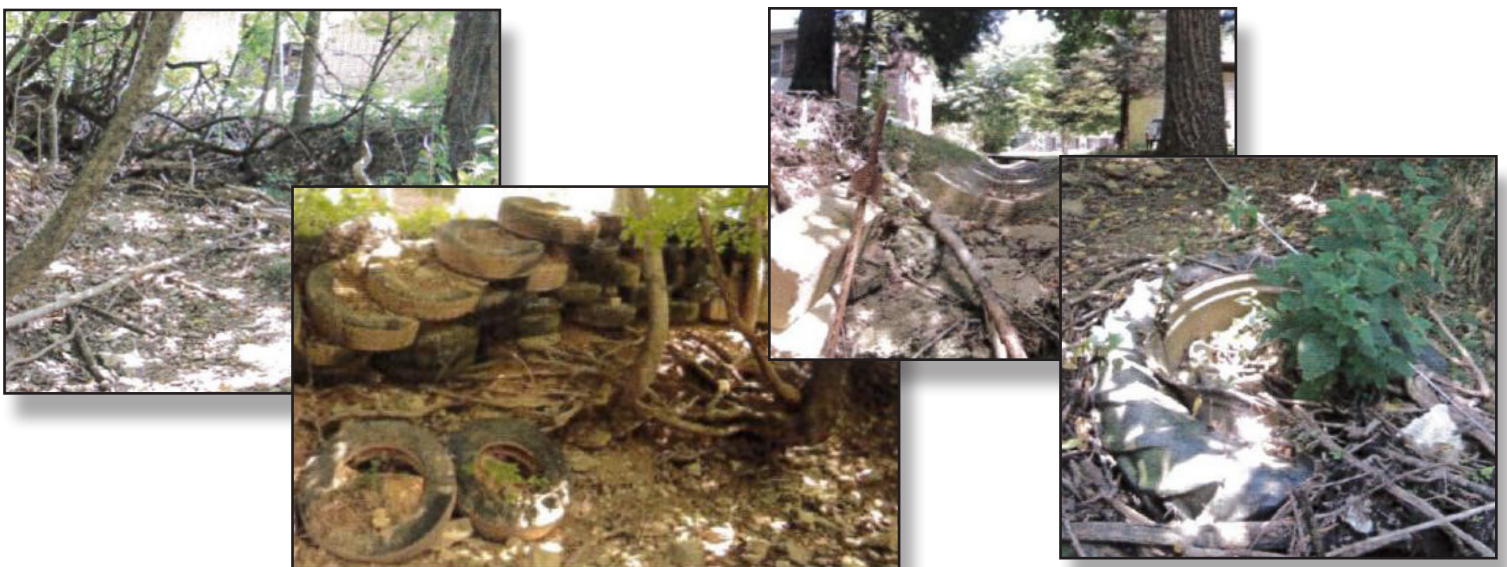
Figure 10. Ballard Court project area. Left to right: Migrating cut bank, tire wall, unprotected concrete swale outfall, debris in the stream bank (photos courtesy of OCFC).
