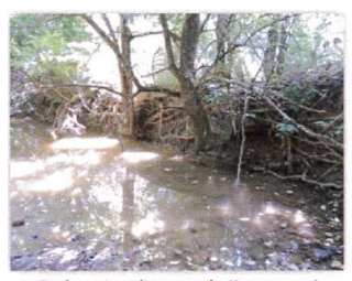
Bank erosion adjacent to the Homeowners' Association Property. The undercut trees are virtually all that remains of the riparian vegetation here.
