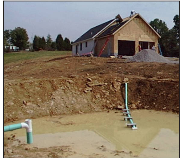
A septic lagoon under construction. It replaces the leach field in the septic system. (Photo credit: KY Dept. for Public Health)
