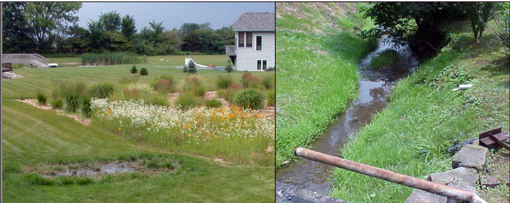
Examples of a failing septic system with surfacing effluent (left, Kellie Hart, UK extension) and a straight pipe (right, US EPA)
