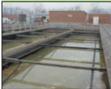
Owensboro wastewater treatment plant
