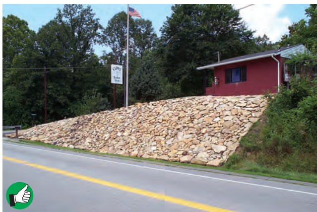
Good slope protection with permanent rock cover. This slope could have been protected with erosion control blankets or mats and seeded for a "softer" look.
