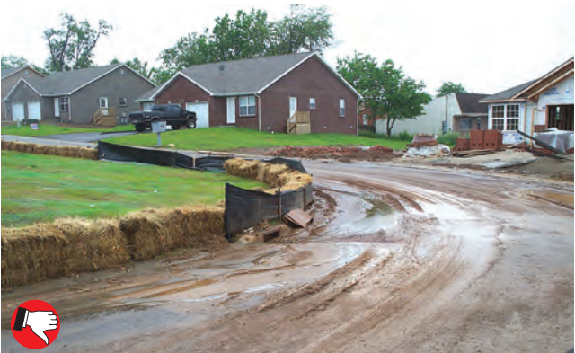
Poor sediment filter installation, no curb inlet protection. Bales alone provide poor protection (note mud on pavement). Very good seed application.
