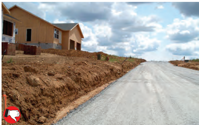
Poor management of bare soil areas on residential construction site. Temporary or permanent seed or mulch must be applied as soon as final grade is achieved.
