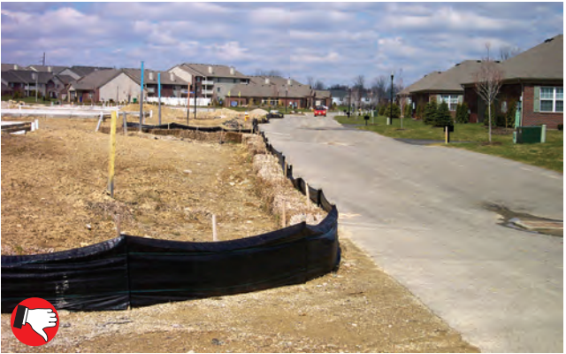
Sediment barrier installed backwards. Silt fence fabric should face bare soil area. Stakes go on downhill side. Straw bales can be used to back up fence on downhill side, but not alone.
