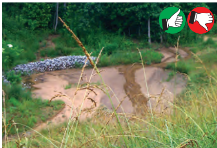
Good sediment trap installation, but poor maintenance has caused trap to fill and bypass to occur. Remove sediment before trap is half full. Make sure containment dike has an overflow notch to control the discharge location.
