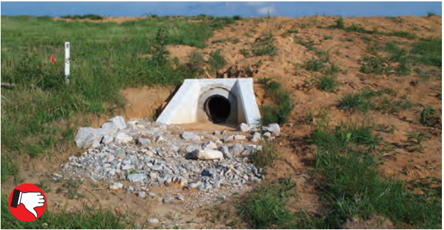
Poor rock apron placement and construction at culvert outlet; poor seeding and slope protection (right side).
