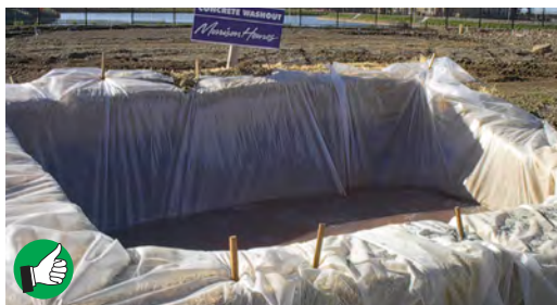
Acceptable containment structure for concrete waste and truck wash water. Make sure that additional structures are available as existing ones are filled.
