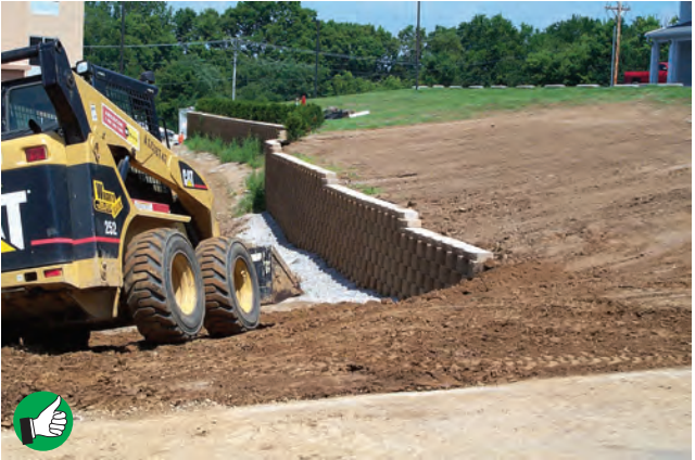
Good use of engineered retaining wall to break up slope. Development site and customer preferences will dictate type of materials used.
