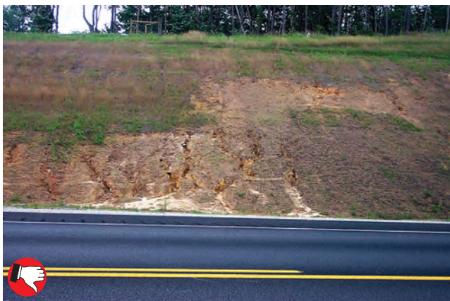
Poor seed establishment on slope. Use erosion control blankets or turf reinforcement mats when slopes are steep (greater than 4:1) and soil quality is poor. Terracing or benching steep slopes also helps.
