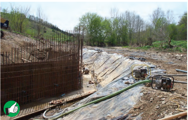
Excellent use of temporary plastic covering during bridge construction to reduce slope erosion. Filter sediment from pump discharges or discharge to protected infiltration area away from waterways.
