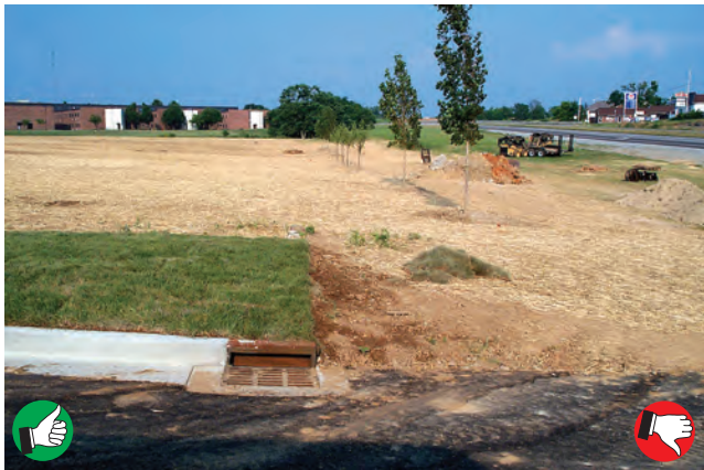
Good mix of sod, seed, and mulch at site of new community center. Note that inlet should be protected by installing a rock or sandbag berm to pond water before it flows into the inlet.
