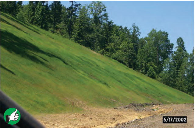
Excellent slope protection with seeding and erosion control blanket. Blankets or mats are required on most projects if slopes are 3:1 or steeper. KYTC requires blankets on all slopes longer than 100 feet if they are 4:1 or steeper.
