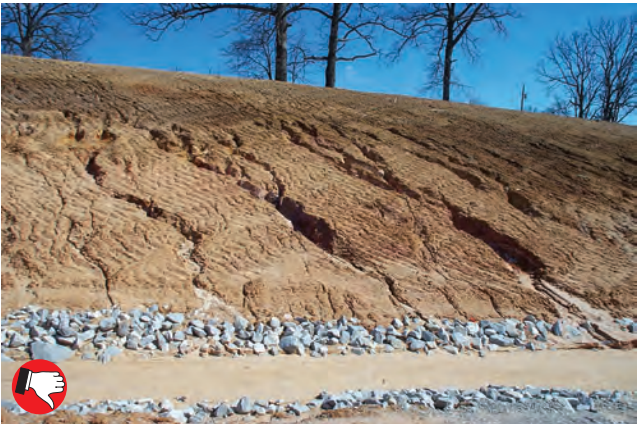
Very poor slope protection. For best results, prepare soil and apply seed with mulch or blanket immediately after reaching final grade.
