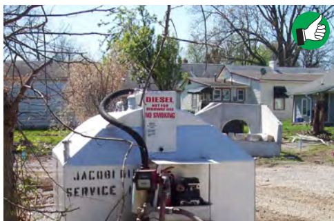
Double wall fuel tanks should be used. Locate them away from ditches, storm drains, and waterways.
