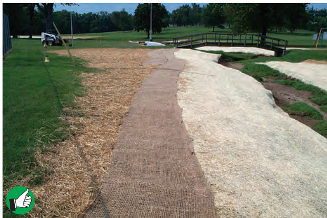
Excellent soil coverage at stream bank stabilization project using hand scattered straw, jute matting, and erosion blanket.
