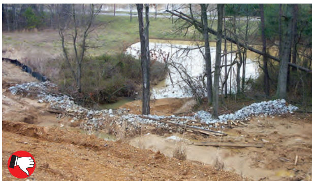
Poor sediment trap construction. Dike is poorly built, without an overflow notch. Placement is too close to pond. No seeding or mulching evident in drainage area.
