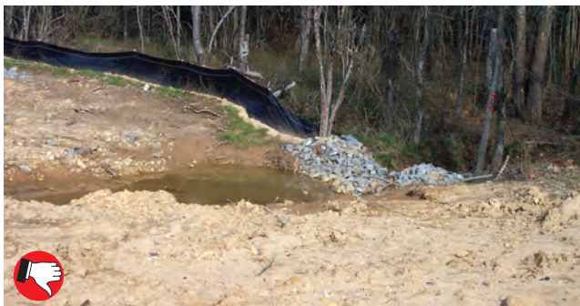
Fair to poor trap installation. Dike overflow notch is too deep; basin is too small. No seed or mulch covering bare soil areas.
