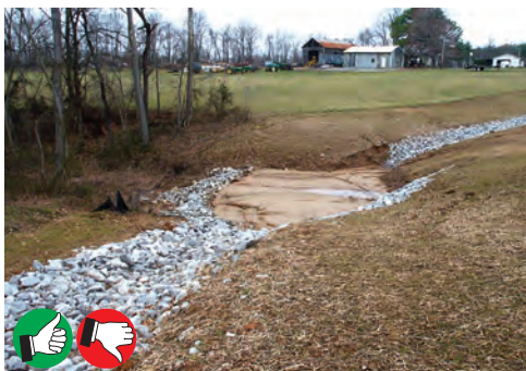
Good trap location; needs cleaning out. Trap might be too small for area drained. Very good channel protection, seeding, and mulching.
