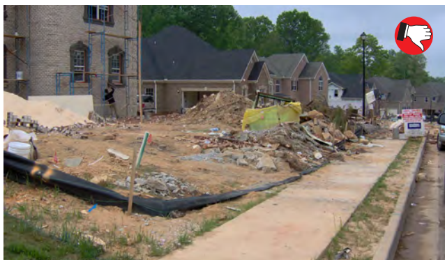
Poor solid waste, silt fencing, and other controls. Failure to control waste and sediment are violations of the KPDES Stormwater Permit.
