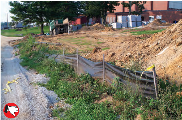
Very poor attention to silt fence maintenance. Fences and other sediment controls must be inspected and repaired weekly; activities should be logged.
