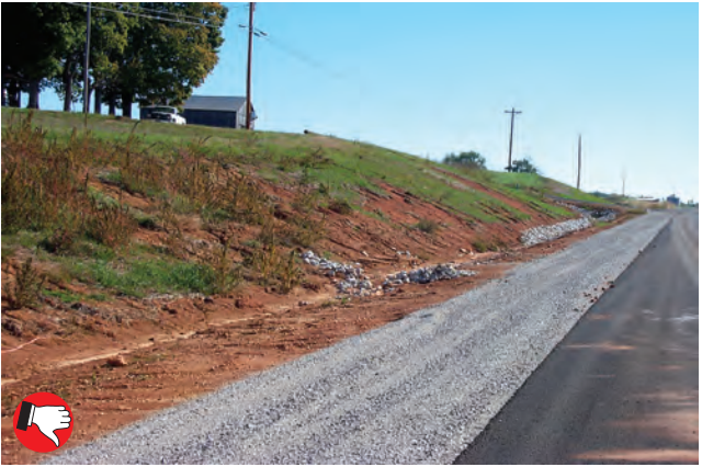
Poor slope protection. Seed has washed away—blankets or mats should have been used. Channel lining is poor. Silt check dam has washed out; more silt checks are needed.
