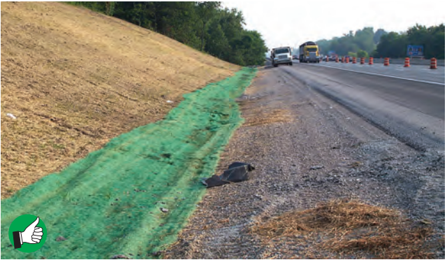
Very good installation of erosion control blanket in seeded ditch below well-mulched slope on highway project.
