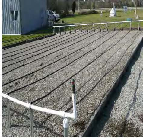
Figure 7. Geoflow Drip Irrigation System
