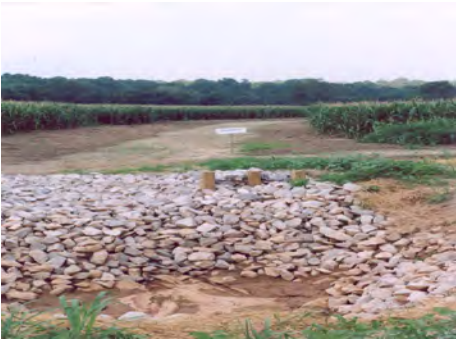
Figure 22. Photograph on the top shows a sinkhole without setback and waterway located in a future corn field. Photograph on the bottom shows the finished setback and waterway construction in the same corn field later in the season.
