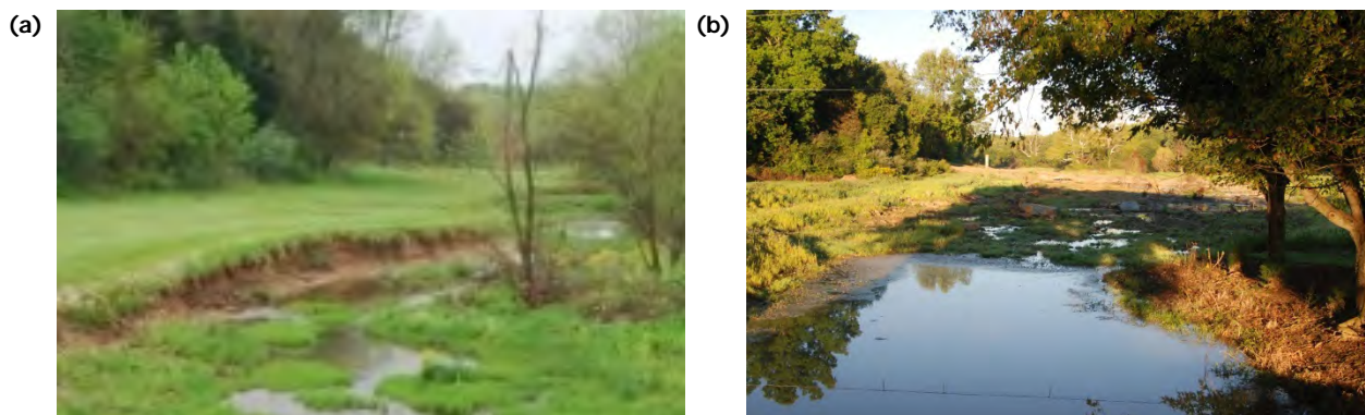
Figure 3.1 South Fork Currys Fork (a) before and (b) after restoration. Bank heights and local sediment supply were dramatically reduced, and in-channel sediment storage potential was increased due to the construction of a wide, frequently-inundated floodplain.
