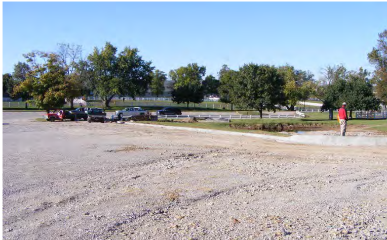
Figure 39. Concrete curbs were installed around the perimeter of the parking lot to direct runoff toward the settling basin
