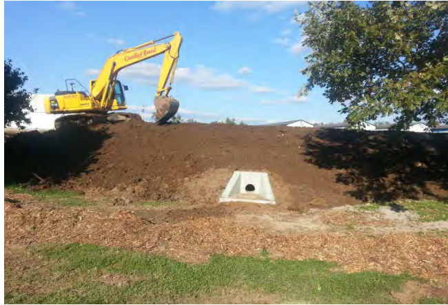
Figure 23. A bioretention pond was installed below an impervious area where horse wash racks and uncovered manure piles are located and labeled with education signage
