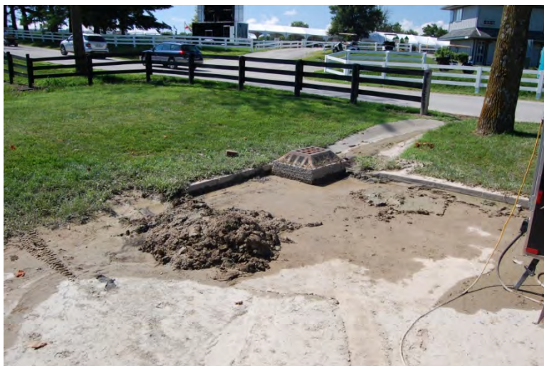
Figure 38. A pervious concrete frame was installed around the storm drain inlet to filter the sand and sediment from runoff and topped with a grate covered in a wire mesh.
