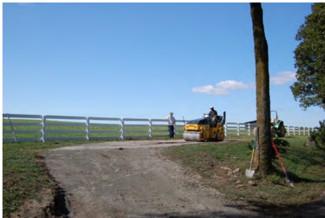
Figure 28. A highly erodible section of the visitor horse trail was paved with soil cement
