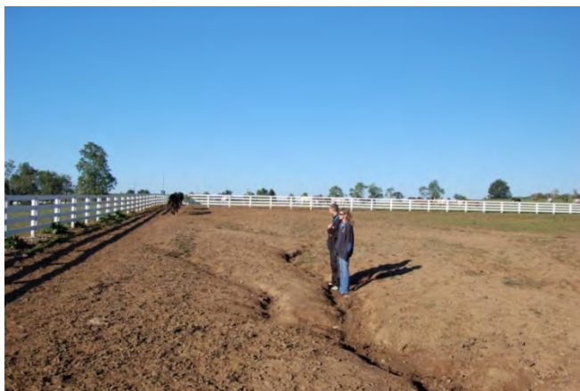
Figure 31. Large gullies flowing toward trail horse paddock
