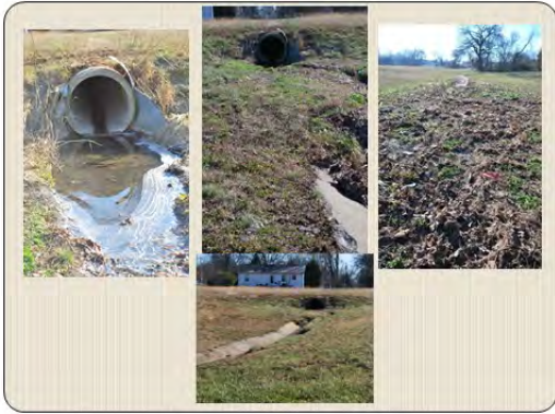
Fig.3: Images showing erosion from velocity and heavy discharge onto site
