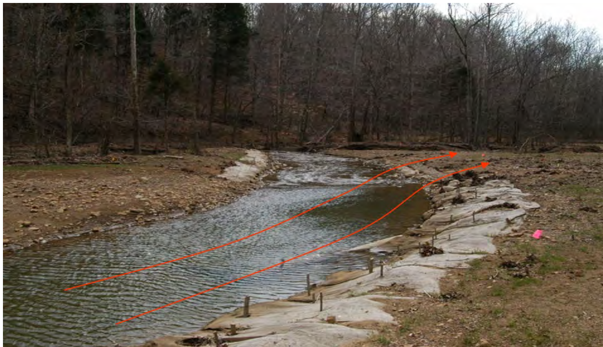
Figure 1 Flow overtops banks as it leaves the bend. Note the erosion control matting is still in place at the toe of the bank downstream of the bend. Ruts have formed in the unvegetated floodplain and on the top of the bank near the flow indication arrows.
