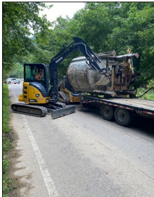
Photo 13: Southeast KY Flooding – Spill Response
