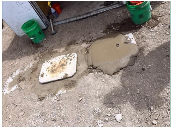
The testing area is on-site, away from the activity. A shed is used to hold the samples for field curing.
