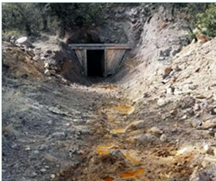
Figure 2: The adit at Lead Queen Mine, pre-remediation. An adit is a horizontal entrance to an underground mine primarily used for de-watering and extraction of minerals during operations.
