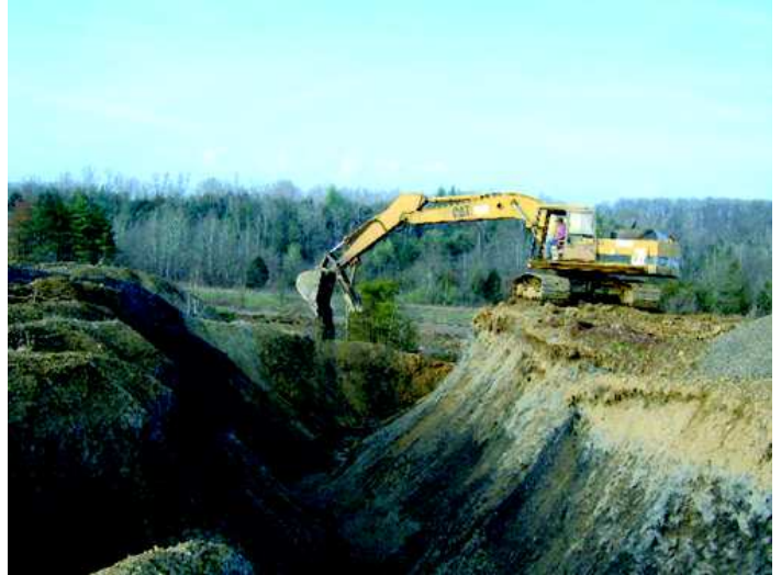
The trackhoe is placing agricultural limestone to neutralize acidic coal wastes prior to grading the gob pile. This preventative treatment measure is being taken because ravines like these often act as conduits for acid water seeps, even after the site is graded.
