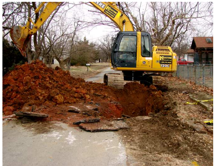
Ute Street Emergency
