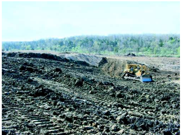
The gob pile will be graded to gentle slopes that minimize erosion and prevent the redevelopment of gullies. The sub-grade coal waste will then be treated with ag-lime and covered with 2 to 3 ft. of good quality glacial-till soil.
