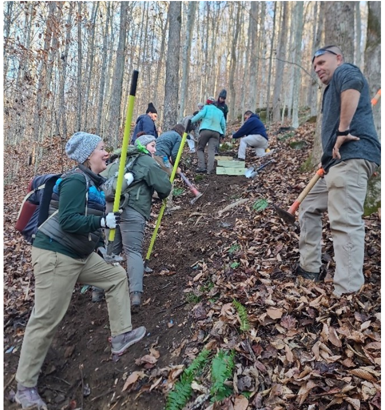
Participants of Trail Workshop help install steps on a steeply graded trail at Buckhorn Lake State Resort Park
