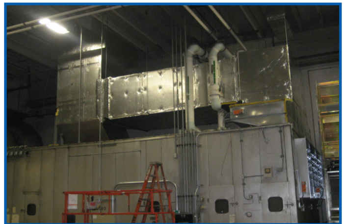
Three air handlers located in production areas were retrofitted with more efficient ductwork using outside air and controls to allow more economical operation.
