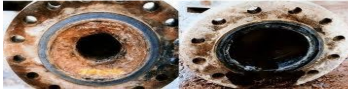
Picture 8-1 Dirty pipe/Clean pipe
