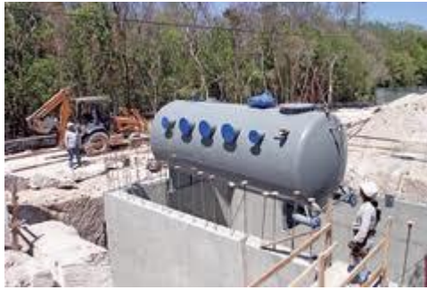
Picture 4-11 Vacuum sewer system tank
