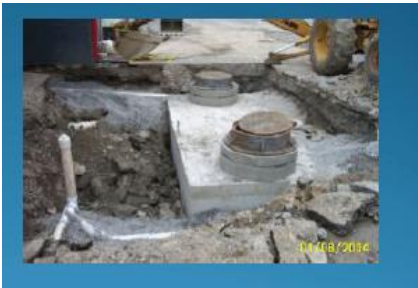
Picture 9-1 grease interceptor
