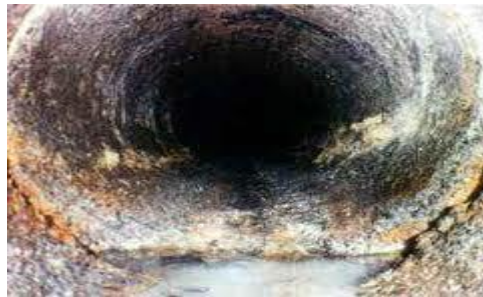
Picture 11-3 Corroded sewer pipe
