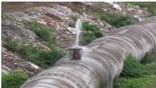
Picture 11-2 Leaking sewer pipe
