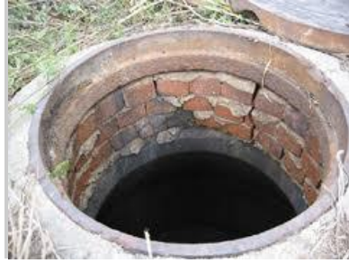
Picture 7-4 deteriorated manhole
