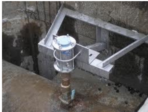
Picture 6-17 Effluent force main valve
