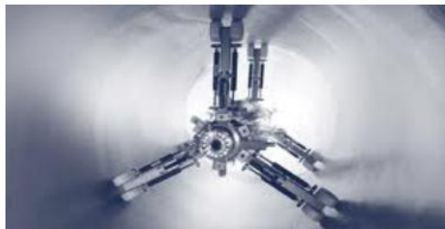
Picture 8-5 CCTV camera in a new sewer line
