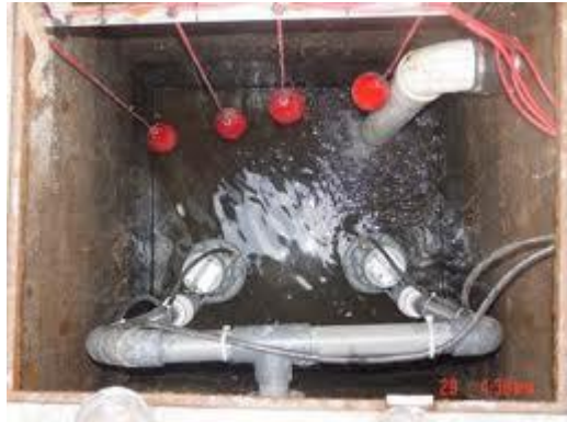
Picture 6-14 Lift station
