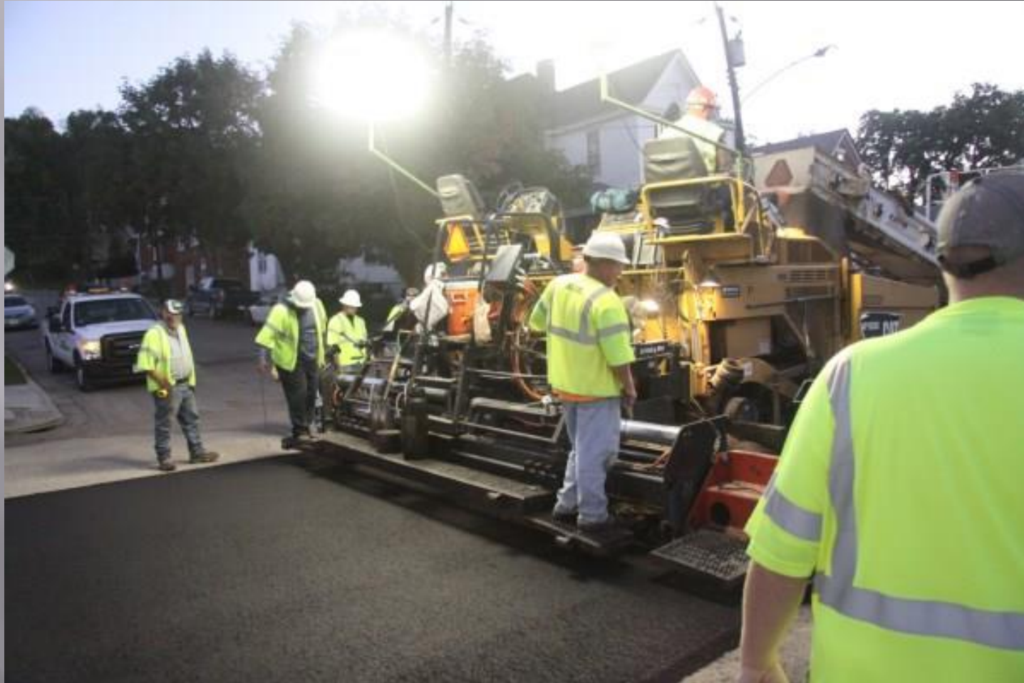
Paving train applying rubberized asphalt looking southwest. Photo by Mark Belshe RPA
