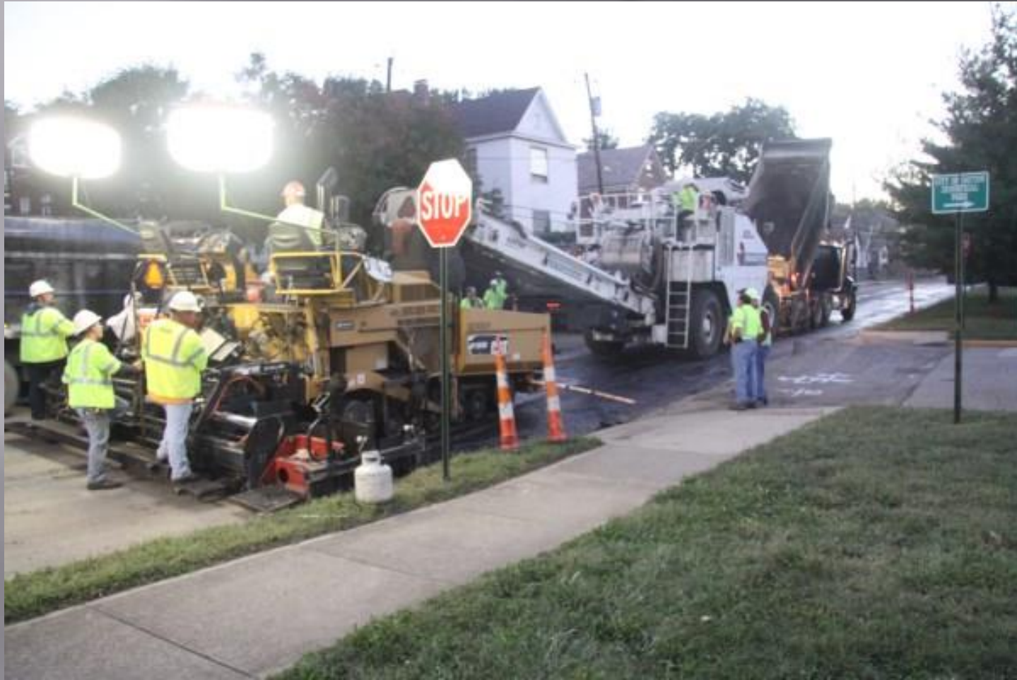
Paving train applying rubberized asphalt looking west. Photo by Mark Belshe RPA
