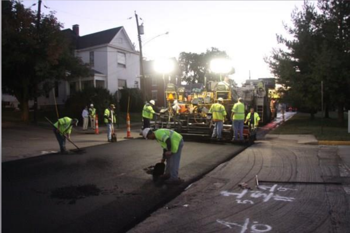
Workers smoothing rubberized asphalt around manholes looking southwest. Photo by Mark Belshe RPA
