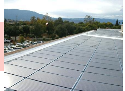
Figure 5. Solar panels reducing energy cost at the water treatment system.
