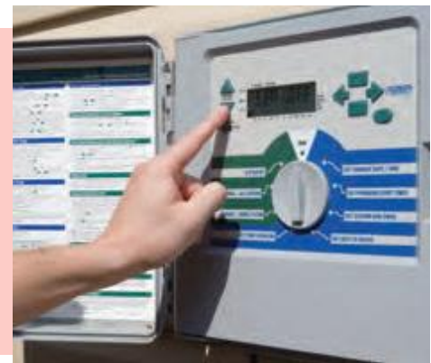
Figure 4. Adjusting a sprinkler system.
