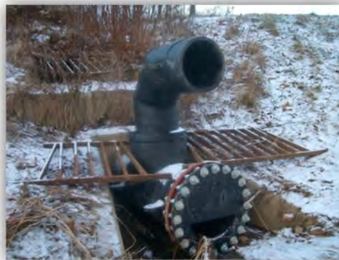
Figure 5-12: Detention basin retrofit outlet structure with bypass, located at Toyota pilot project in Burlington, KY (Photo by Rajib Sinha)
