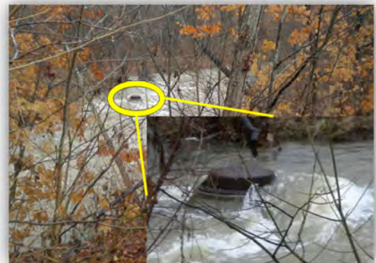
Figure 4-5: Streams widen and destroy public infrastructure
