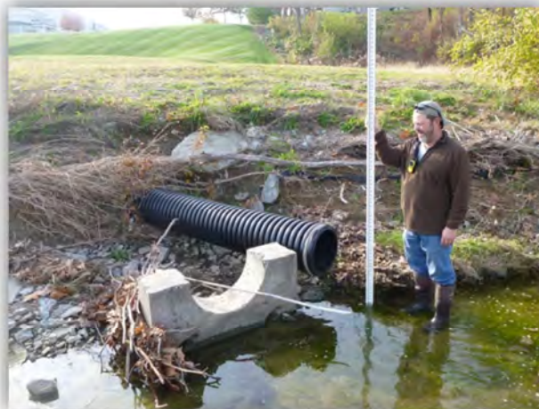
Figure 4-11: Storm sewer infrastructure at Site SFG 5.3-DS compromised by erosive, urban flow regime
