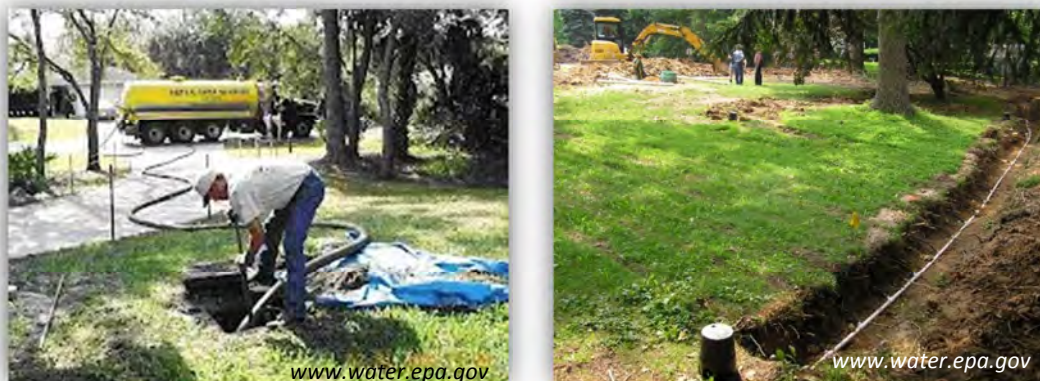
Figure 5-5: Onsite Wastewater Treatment BMPs: Maintenance/septic pumping are routine procedures (left); Placement of the septic system can impact the maintenance (right)
