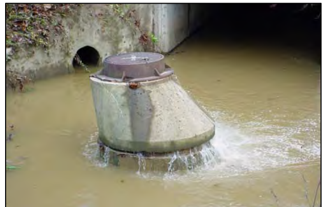
Sanitary Sewer Overflow on Whitley Branch
