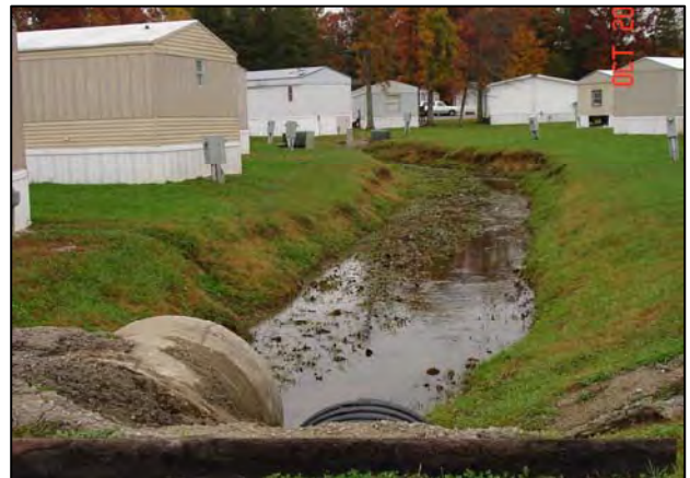
Channelized Section of Sampson Branch (Little Laurel Subwatershed) with Indications of Bank Erosion
