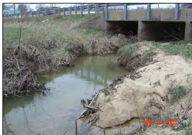
Heavy Sedimentation and Bar Formation
